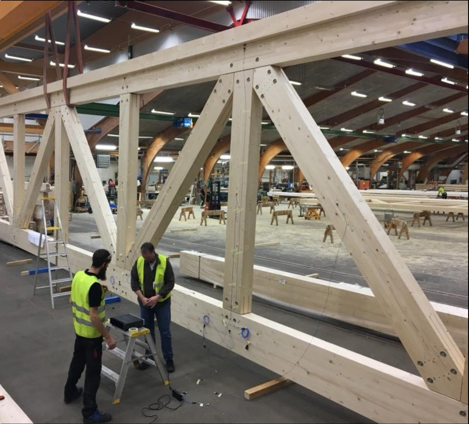
Moelven Töreboda AB. Testings on a glulam truss, factory of the company.
