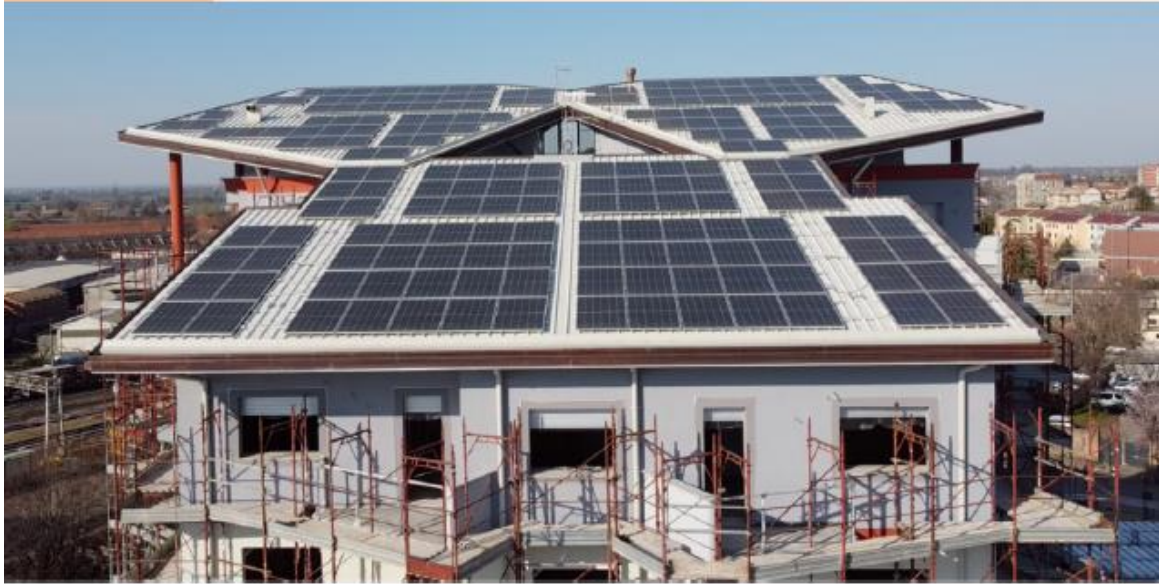
Figure 22 - Photovoltaic system on the roof pitch of the 'Ecocity' building in Tortona (AL)
