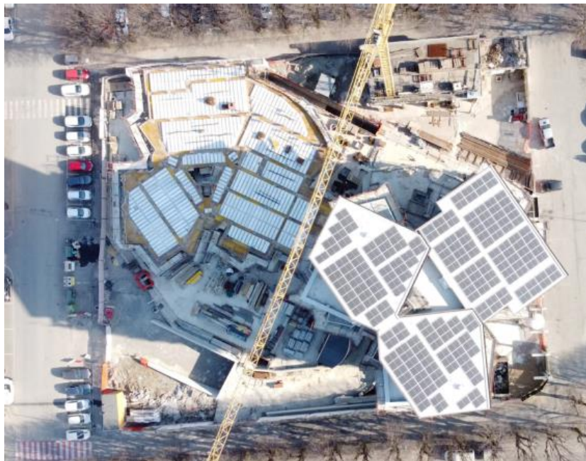
Figure 23 - Construction of the twin buildings that make up the 'Ecocity' complex in Tortona (AL)
