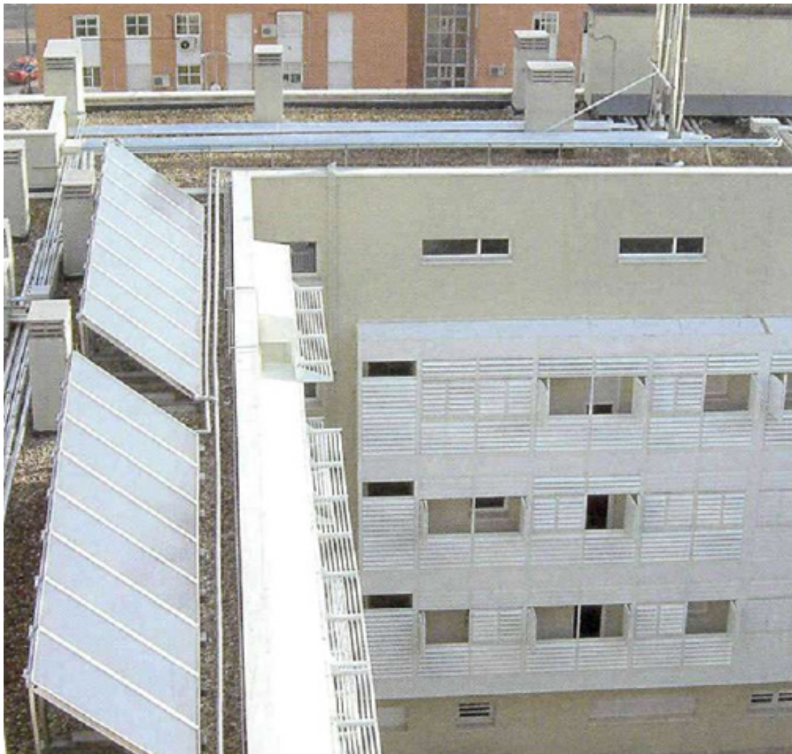
Figure 22: Roof elevation with south facing solar collectors; shading on west facade (courtyard) provided with folding shutters with adjustable louvers
