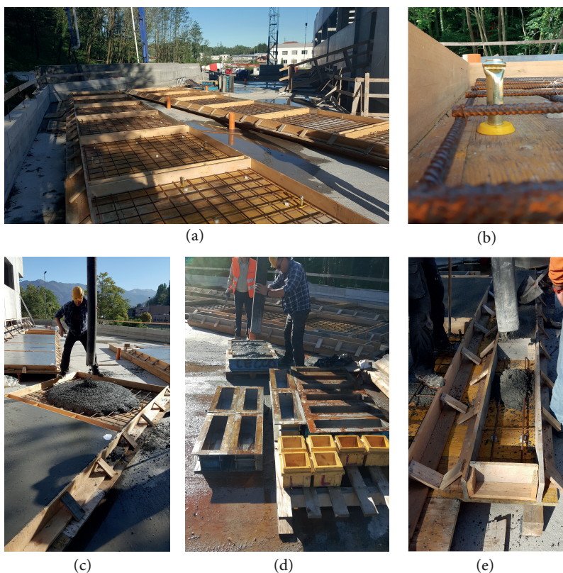
Figure 3.5: (a) The job-site (b) placement of the anchorage device (c) casting of the plates (d) prismatic beams and cubes for compressive strength measurement (e) casting of the shallow beams.
