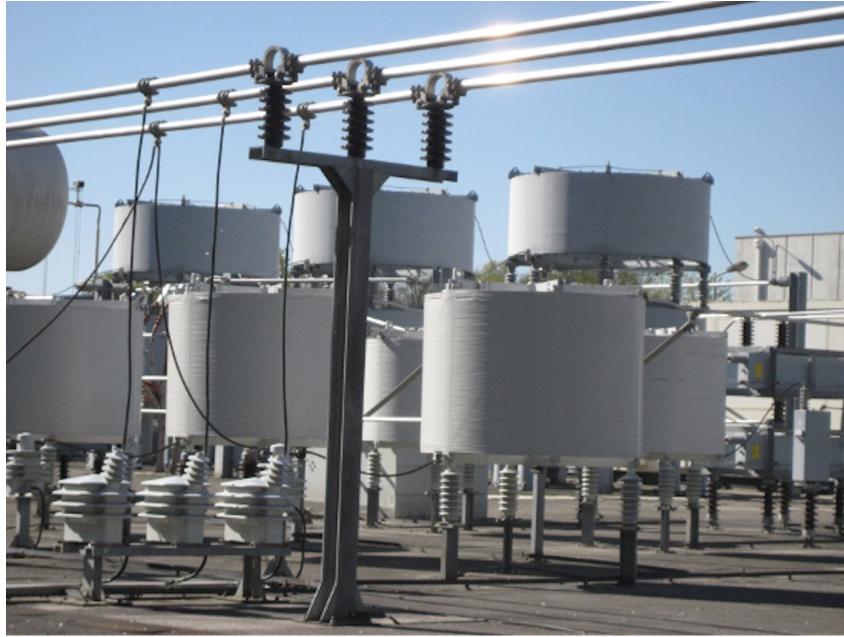
Figure 2.7: The SVC installation affected by the hardware failure. (Image credit: CERN)
