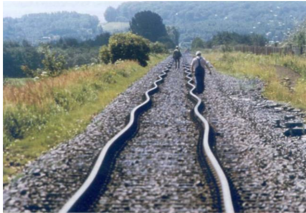
Figure 5-10: Deformation of the rails due to hunting
