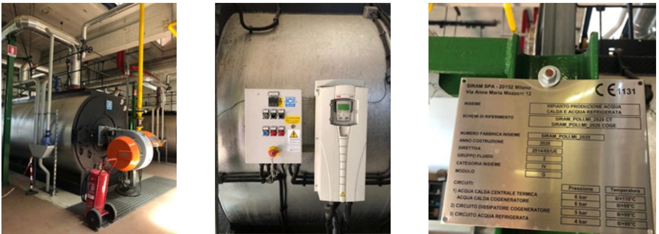
Figure 2-4: Primary system station boilers
