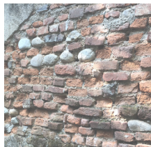
Enclosures in poor condition
