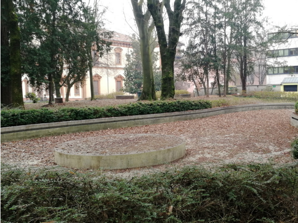
Figure 8. The pond is a hard-paved area that has been abandoned for a long time.
