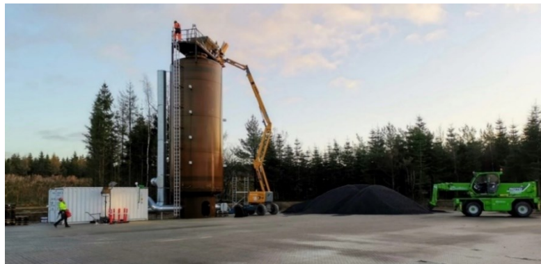
Fig. 2.12: Full-scale reservoir installed at Company HQ, shown during stone-filling experiments (2020)
