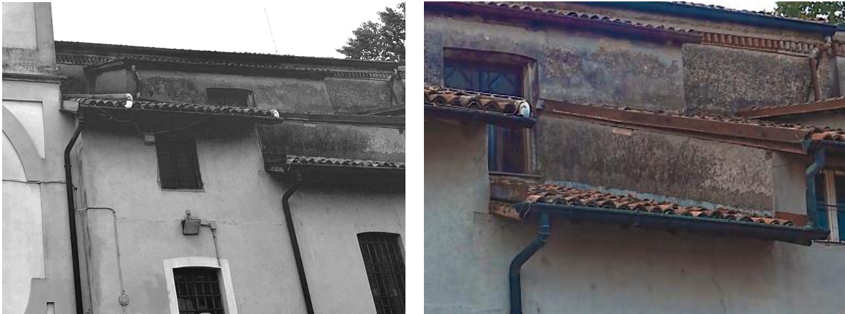
Figure 13 – External Walls Defects
