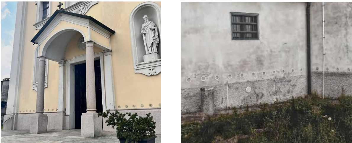
Figure 12 – Conservation through humidity reduction systems
