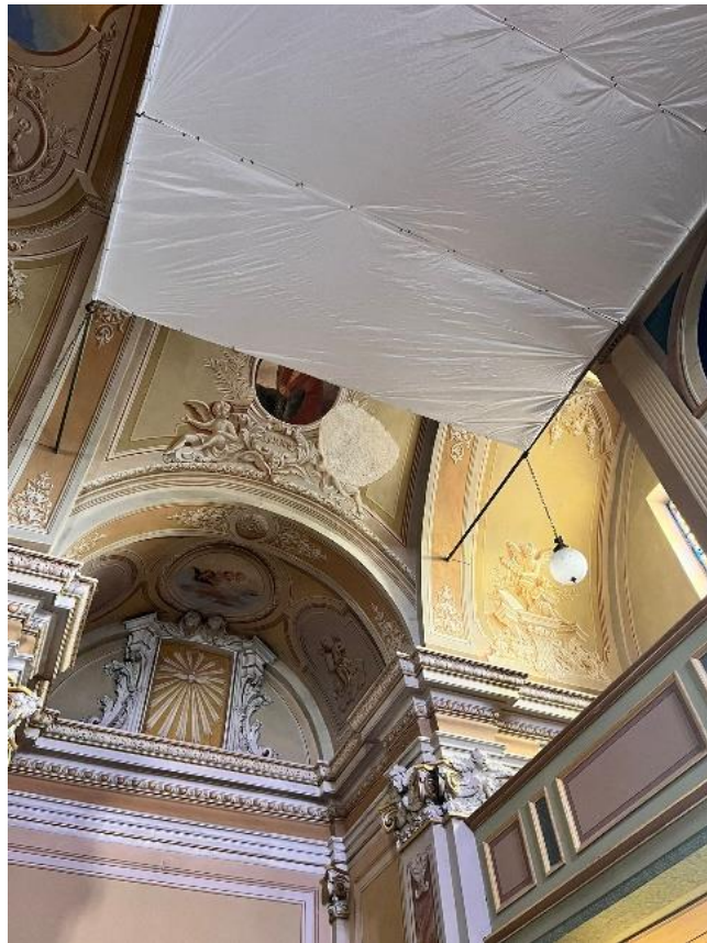
Figure 14 - Protection against plaster detachment
