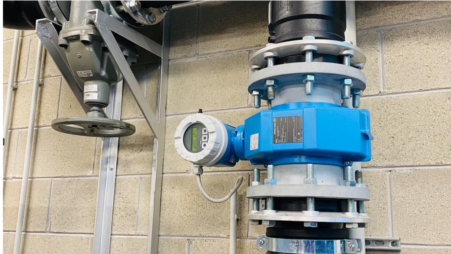
Figure 2-9 Guillotine valve and flow meter
