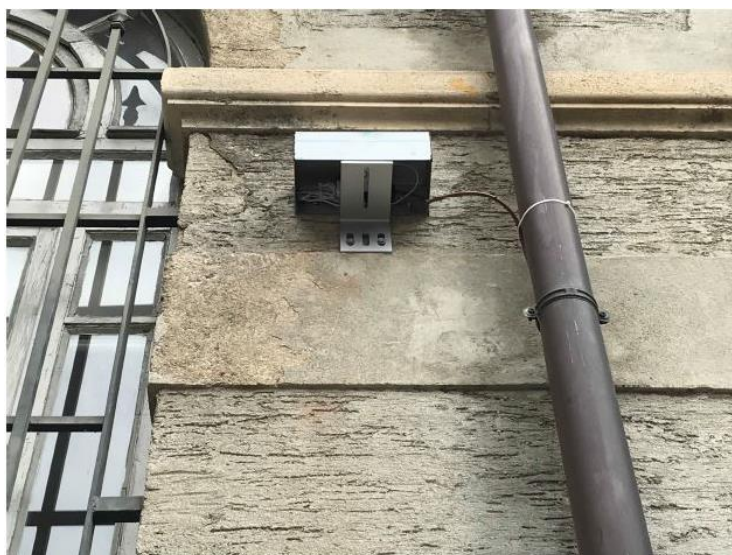
Figure 31: Externally positioned sensor of Green panel installed on Building 9
