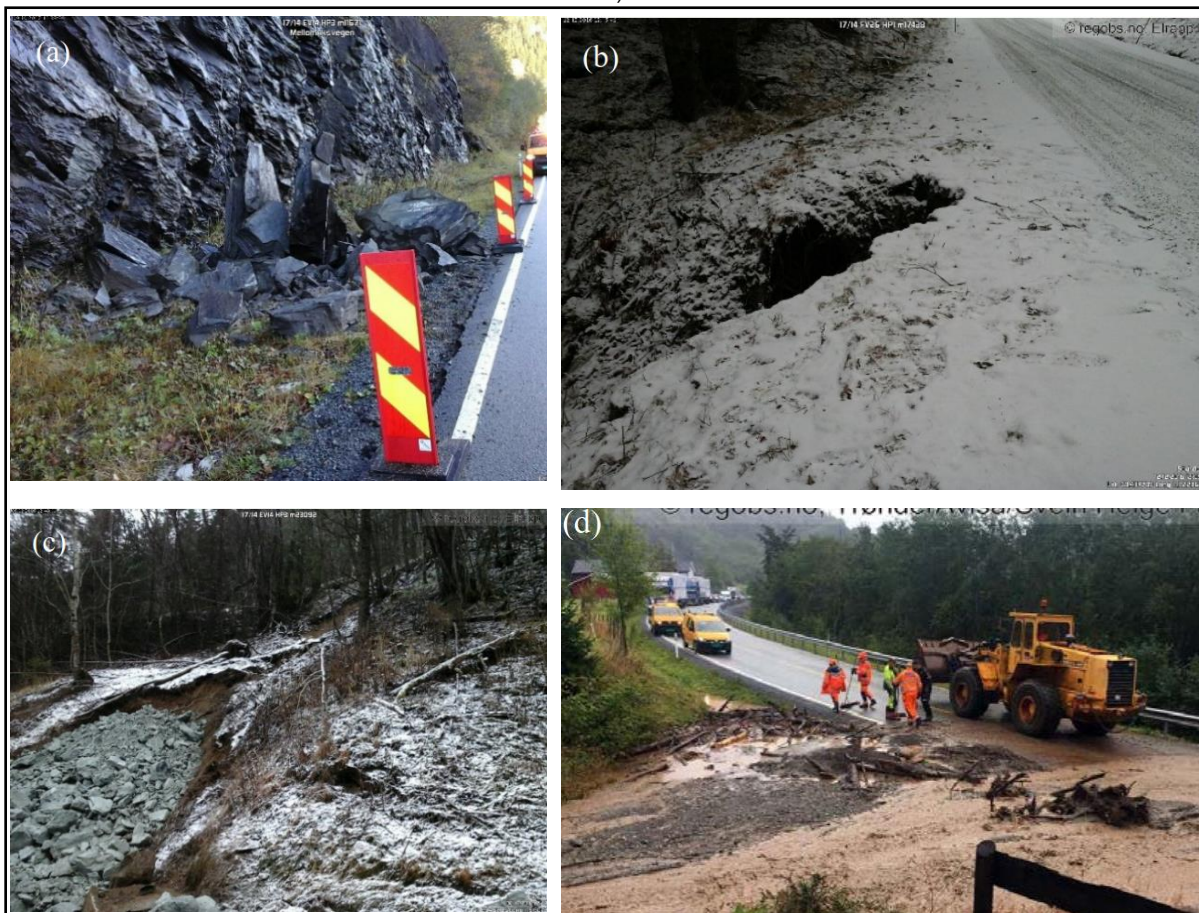
Figure 7. Previous landslide occurred along the road E-14, rockfall (a), soil slides along the road(b), debris slide(c), debris flow(d) (Depina & Oguz, 2021))
