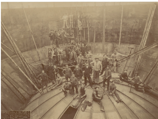
Figure 4.2.r Photo of the potable water tank being installed inside the east tower. 1893. Document in the Civic Photographic Archive (Milan).
