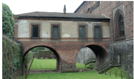
Figure 4.2.e "Ponticella" of Ludovico il Moro, located on the east side of the castle.
