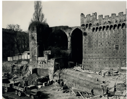
Figure 4.2.s Work in progress at the Rivellino di Santo Spirito. March 1961. Photo from the website http://metromilano.biblio.arc.usi.ch/ .
