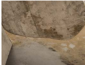
Figure 32. Reinforced concrete structure, Magazine 7 Note. Interior view of a plastered reinforced concrete structure with areas of detachment revealing the underlying concrete.
