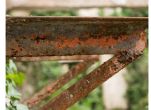
Figure 34. Corroded steel support element, Magazine 5 Note. Corroded steel support element, likely part of a secondary structural addition, with visible material degradation.
