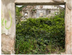
Figure 40. Vegetation growth, Magazine 1, interior space Note. Uncontrolled vegetation growing inside the structure due to the absence of the roof, indicating advanced exposure to weather and lack of maintenance.
