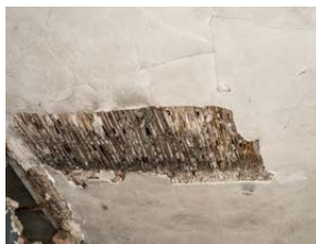
Figure 33. Reinforced concrete ceiling with exposed reinforcement, Magazine 7 Note. Area of concrete cover loss with exposed and corroded reinforcement.
