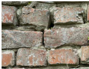
Figure 30. Brick wall, later addition Note. Inconsistent mortar joints, indicating later repair or infill intervention.
