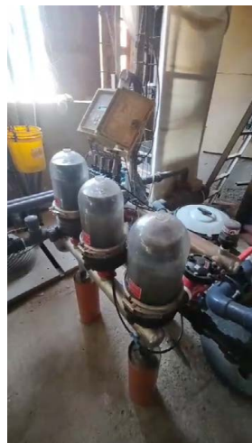
Photo F – The water undergoes filtration through a system called Spin Clean.
