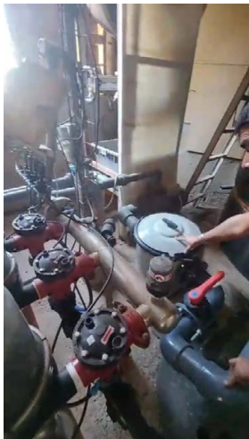
Photo E – The greywater exiting the storage tank and passes through a hair filter to remove coarse debris before entering the main filtration system
