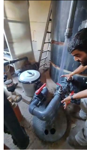
Photo D – Greywater exiting the storage tank.
