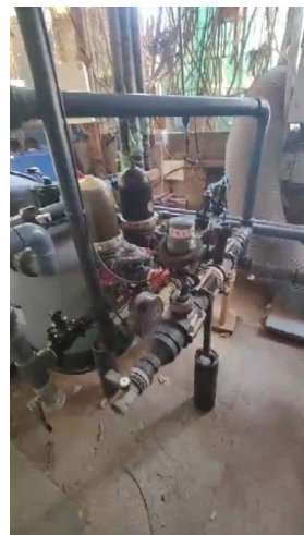
Photo G – The water passes through a sand filter and is then used for irrigation at a pressure of 3.5 atmospheres.
