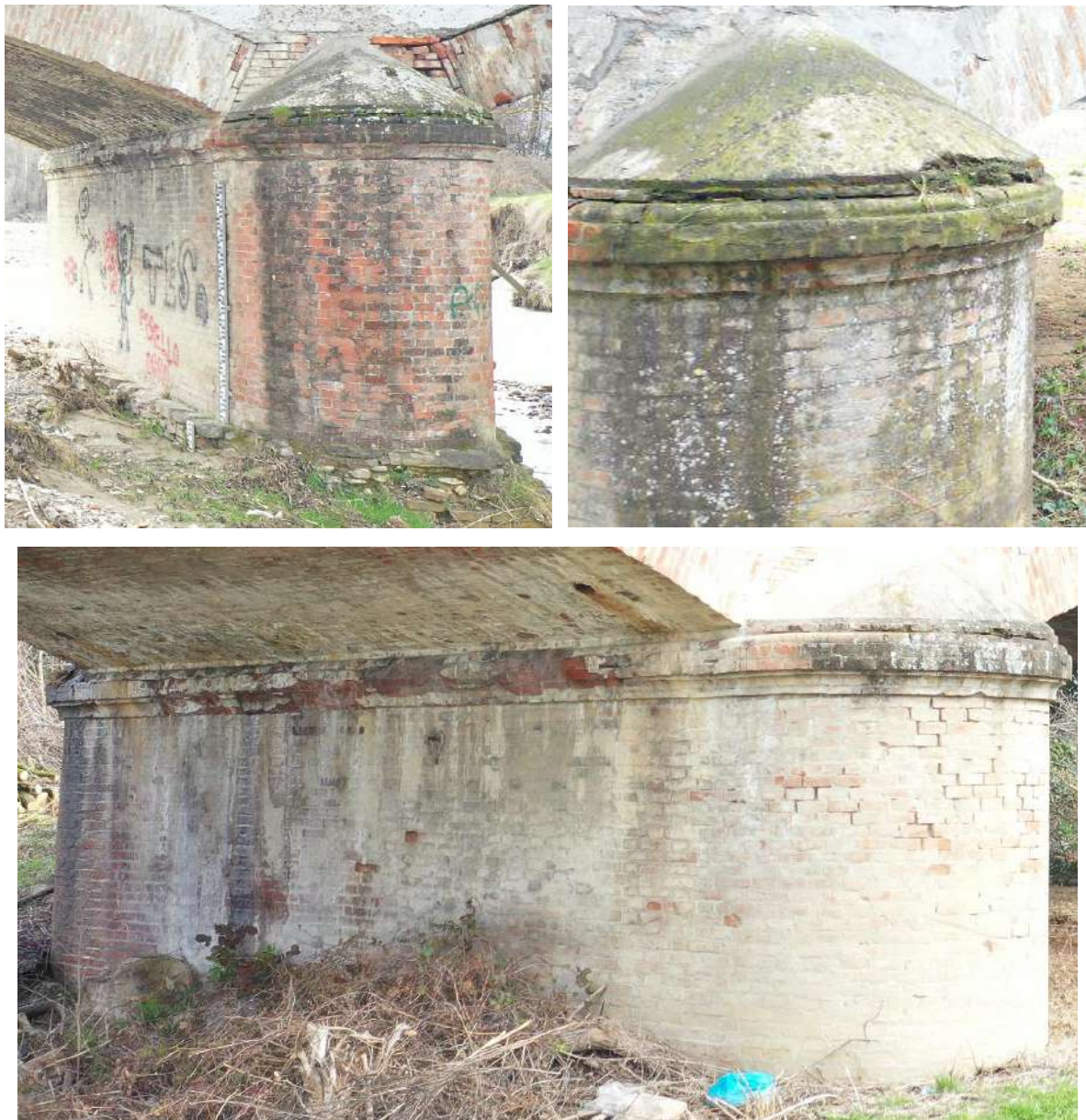
Figure 3.3: Signs of material degradation in the piers.
