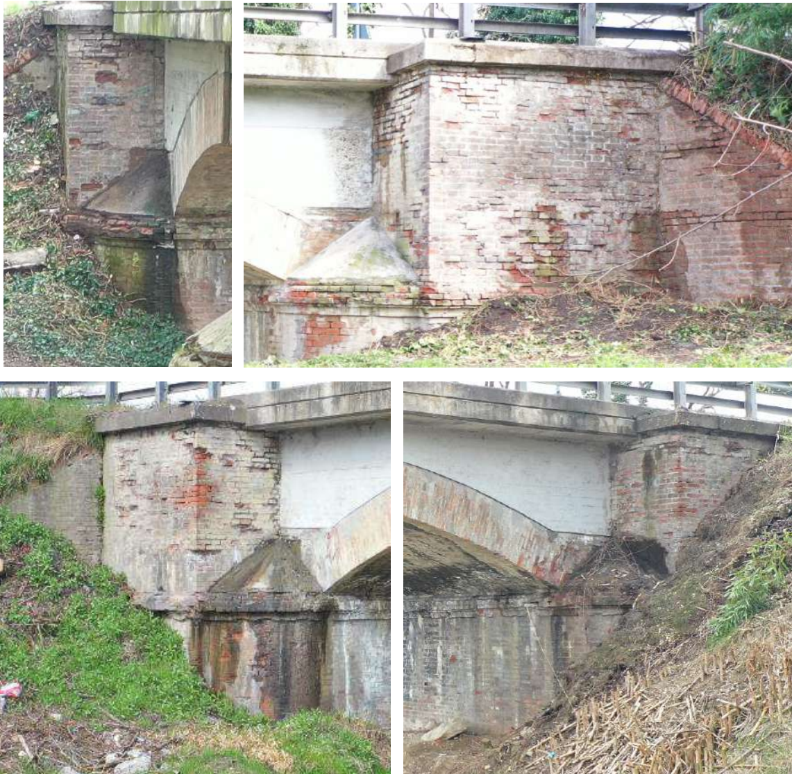
Figure 3.5: Invasion of soil and vegetation and signs of material deterioration of the abutment.
