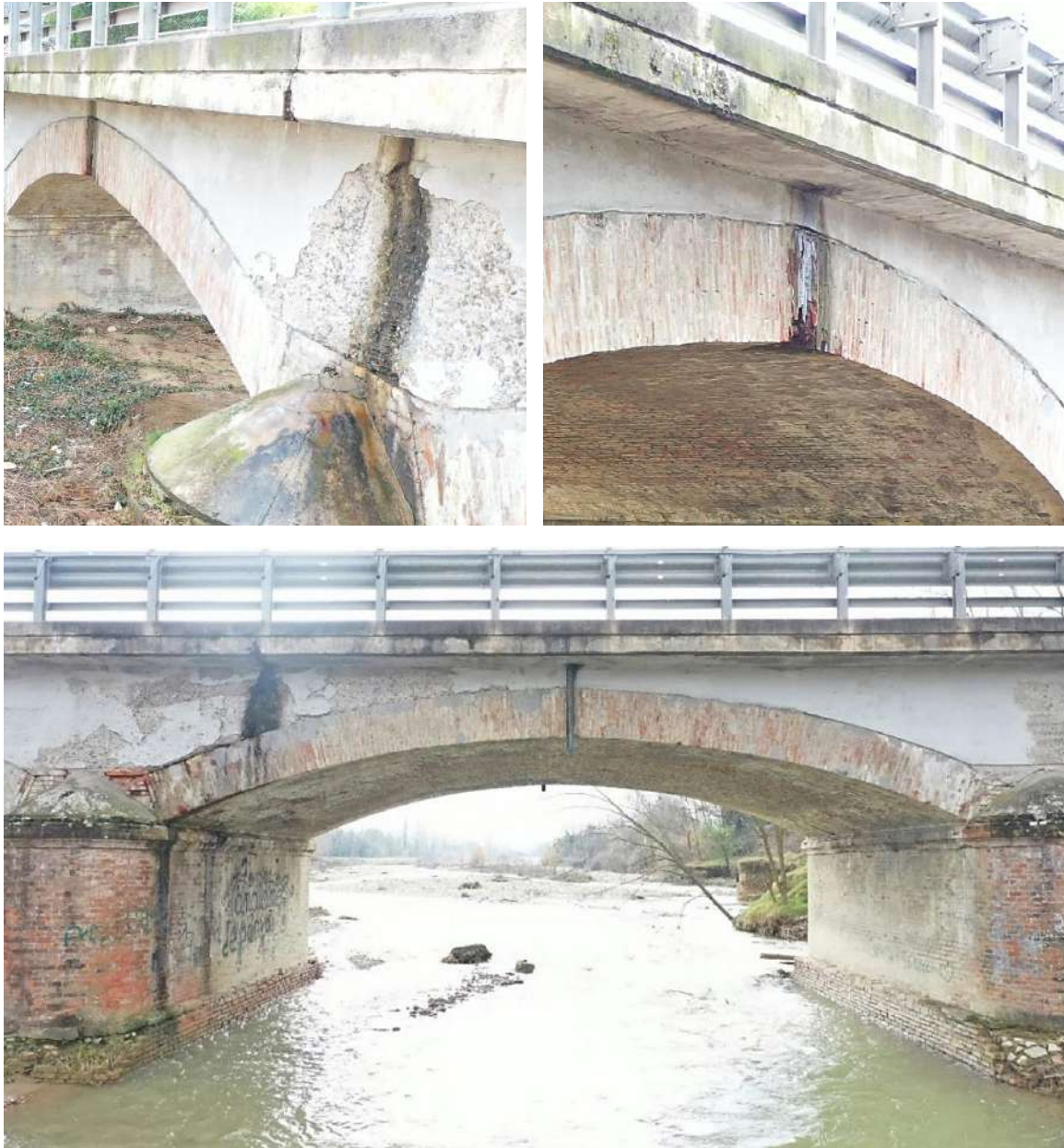
Figure 3.4: Water seepage and concrete spalling in the spandrel walls.
