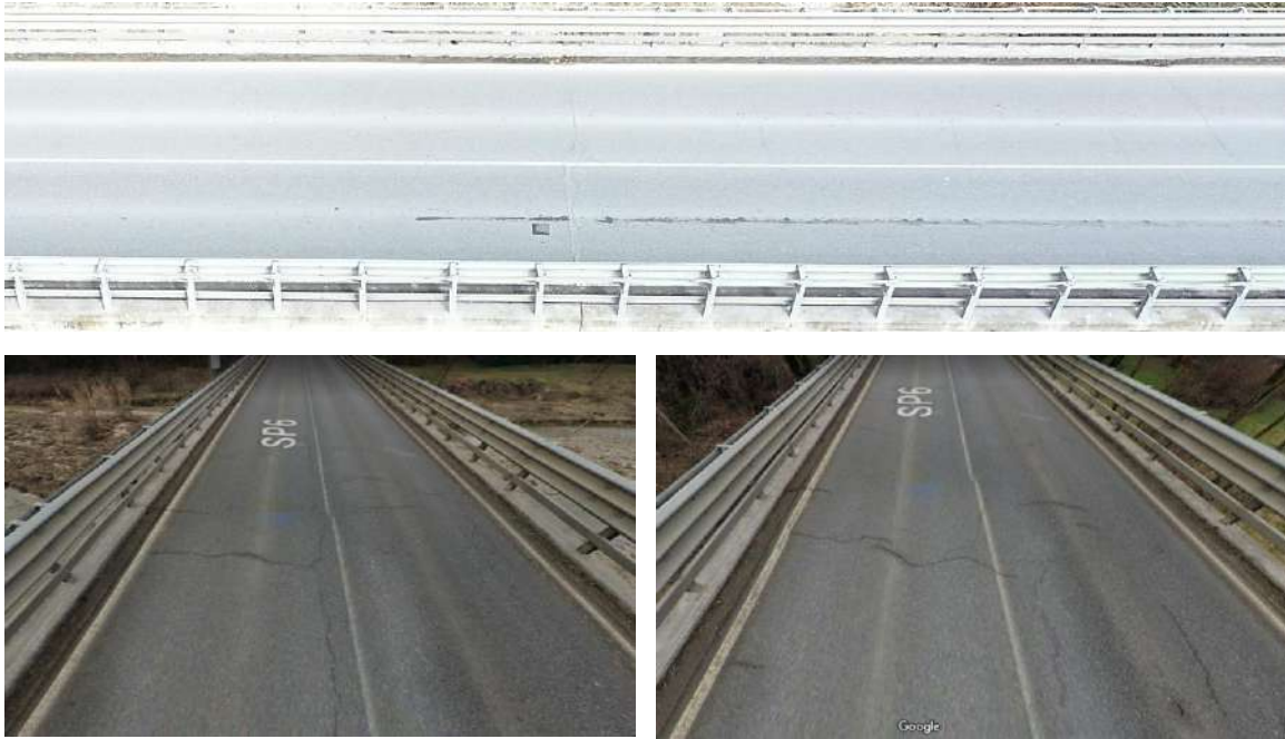
Figure 3.6: Superficial cracks in the concrete decks. Font: Google Maps.
