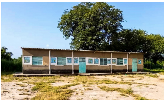
Fig. 1.29 - Abandoned school @Balouo Salo
