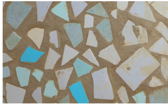
Broken tiles @Balouo Salo
