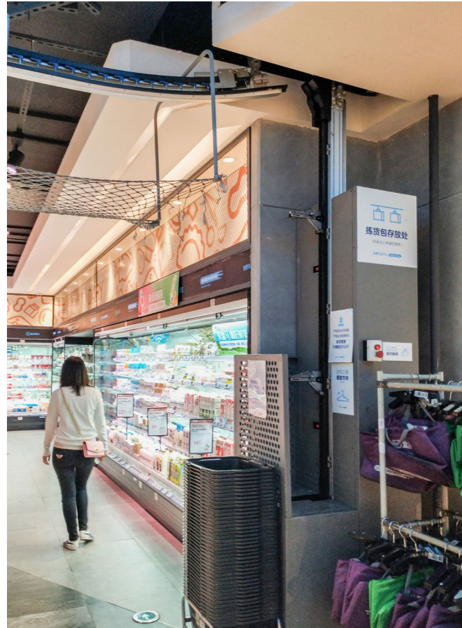
Image 3.15 When the employee finds all the products on the online order, the picking bag will be hung on the transfer point, and the transfer point will transfer the picking bag to the warehouse through the track on the ceiling.
