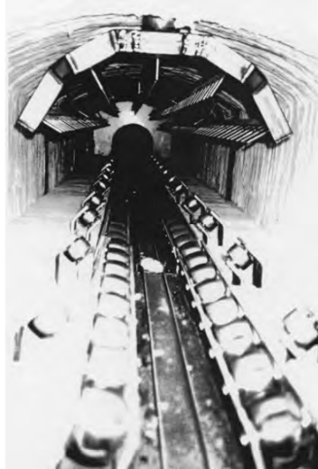
Figure 1.9 Furnace tunnel of a gas-fired furnace with nozzle boxes and nozzles for heating the billets
