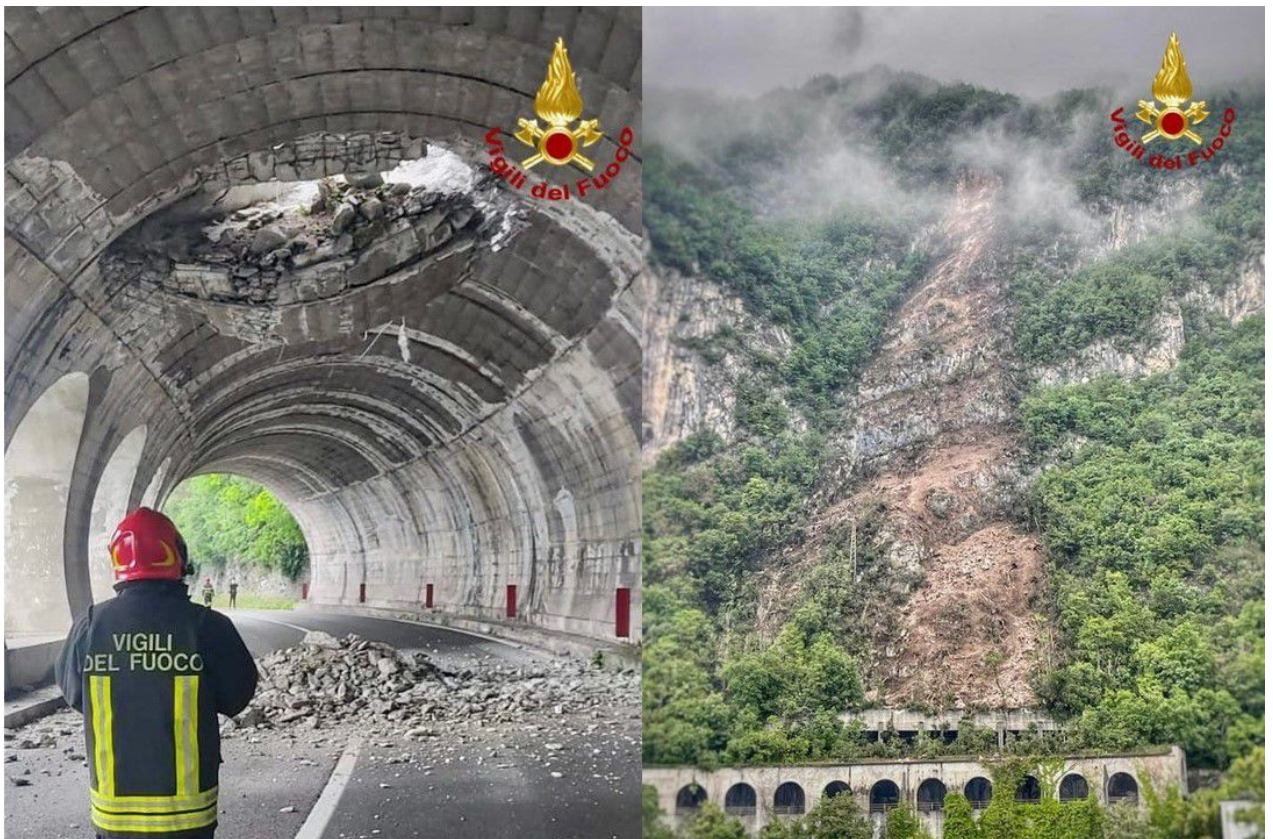
Figure 1.8: Debris flow that broke through the structure of the Fiumelatte road and railway tunnel in Varenna, Italy, (2023)
