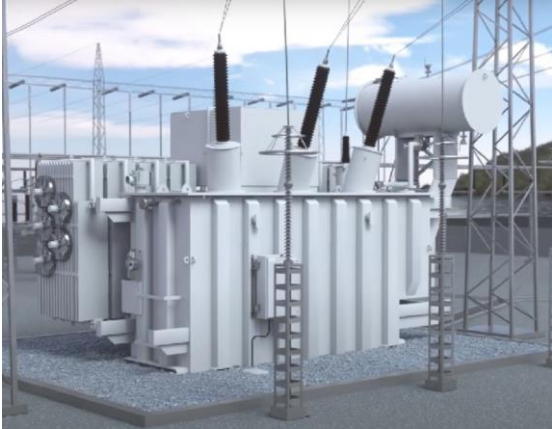
Figure 6 – Distribution transformer tank
