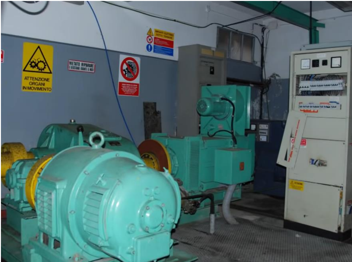
Figure 2.7 The cableway motor winch in the downstream station.
