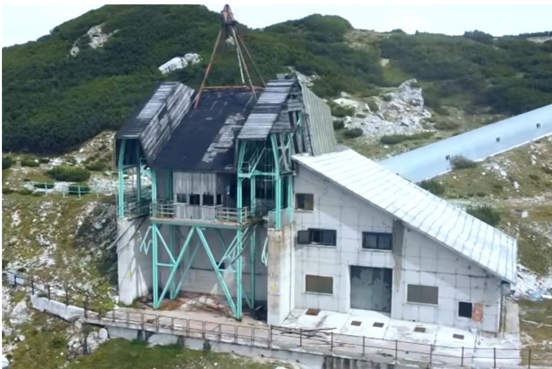
Figure 2.5 Upstream station of Monte Scinauz Cableway.
