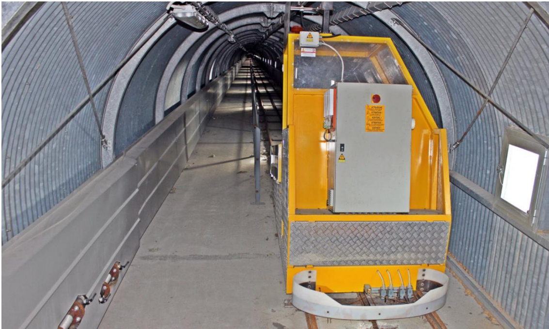
Figure 2.11 The galvanized metal sheet tunnel with the inclined rack rail and the carriage system.
