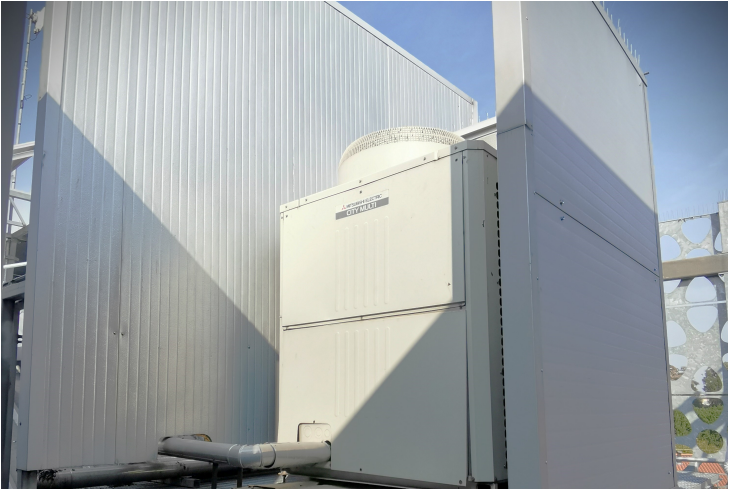
Figure 2.11: Outdoor unit PURY from Mitsubishi installed in the last floor.
