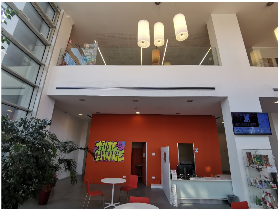
Figure 4.10: Another photo of the diffuser in the atrium.
