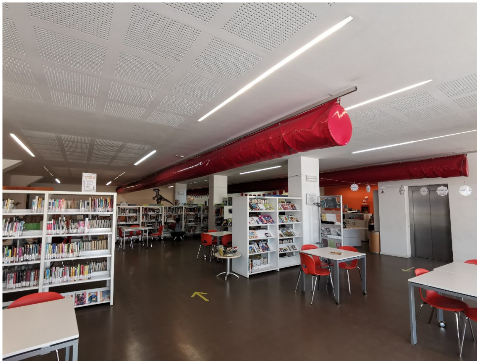
Figure 4.11: Air diffuser at first floor space.
