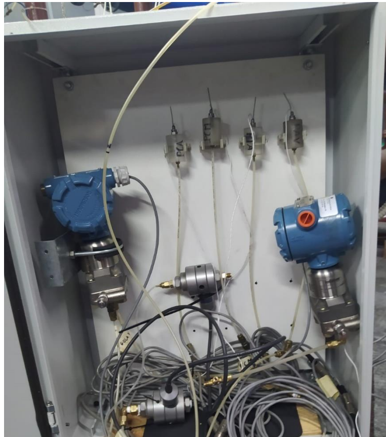
Figure 29 - Pressure transducers' casing
