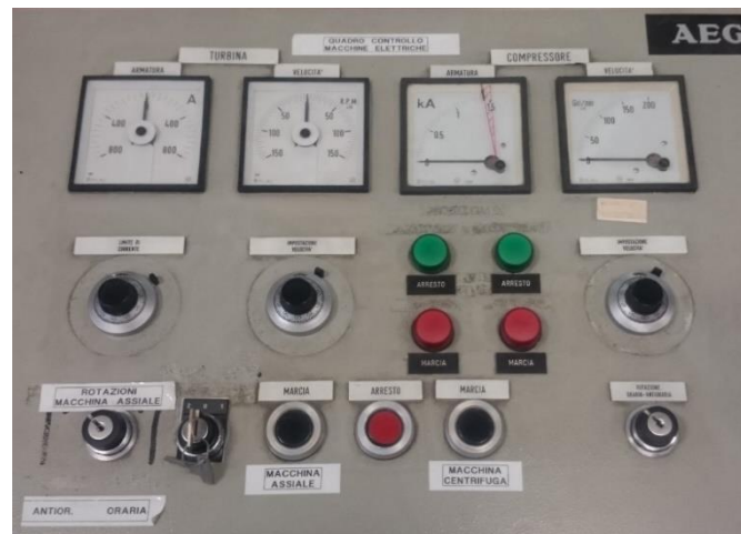
Figure 11 - Control Pulpit of the Test Bench
