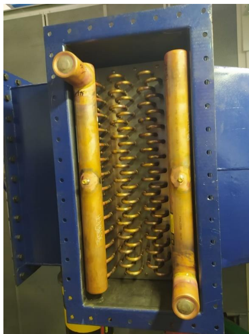
Figure 23 - Heat Exchanger in its casing
