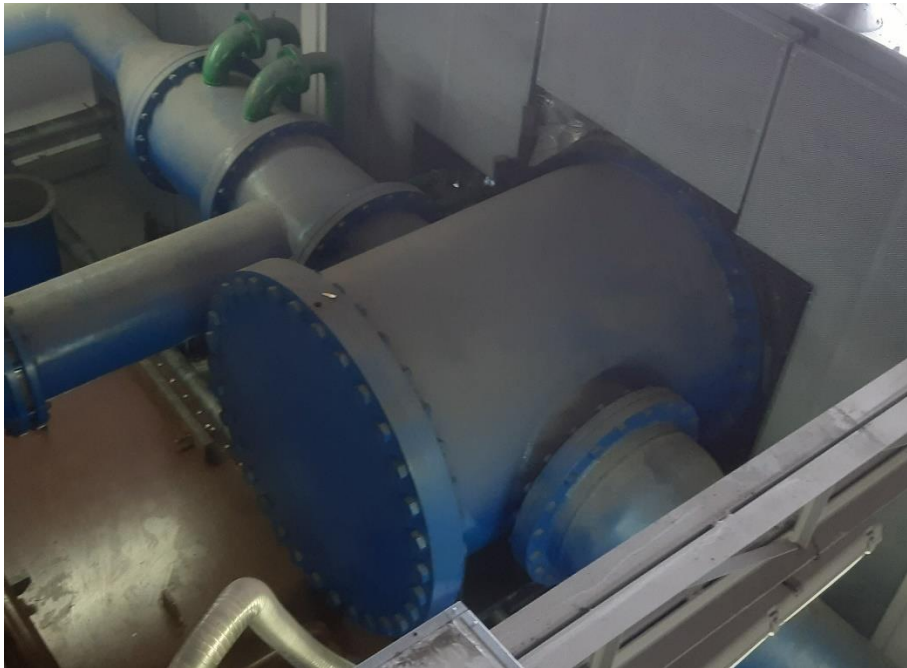
Figure 9 - The two heat exchangers
