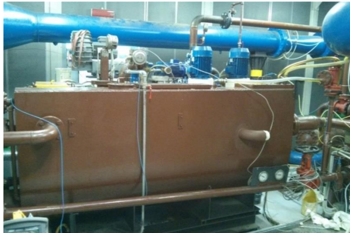
Figure 8 - Picture of the oil tank and the pumping system
