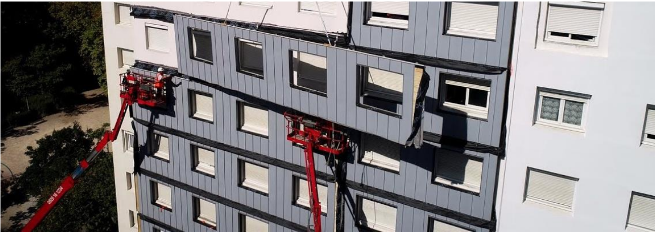
Figure 13 Installation of industrialized panels for the social building owned by Est Métropole Habitat near Lyon
