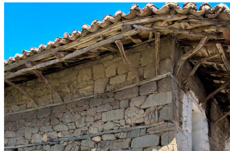
Figure 23 - An interesting roof cornice with support struts made of nailed branches in a traditional building. (CELIM, Albania)
