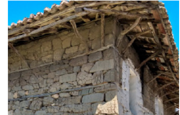
Figure 6 - An interesting roof cornice with support struts made of nailed branches in a traditional building in Nartë.
