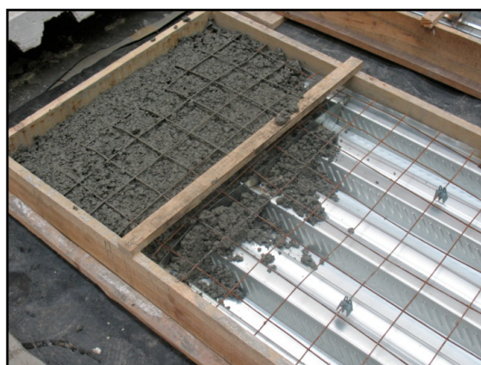
Figure 16 - LWC ponding over profiled sheet
