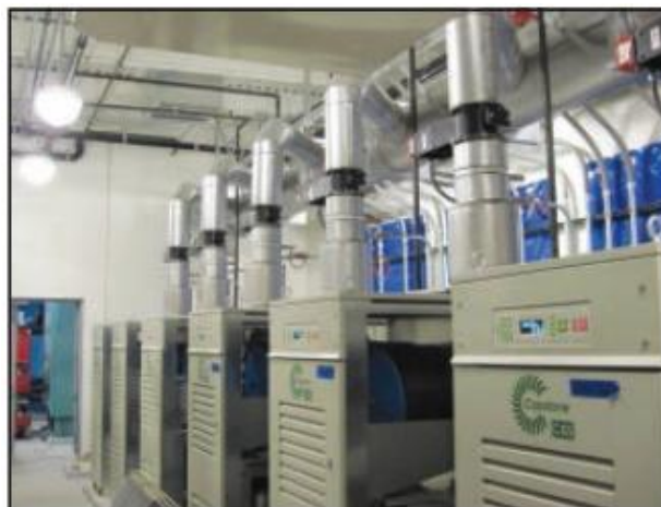
Fig 5.8: Key components of the US$12.4 million Green Data Center at Syracuse University are 12 patented Capstone Hybrid UPS Micro Turbines from Capstone Turbine that provide power to the entire facility. [3]
