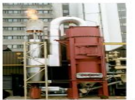
Figure 5.2: Gasifier at Vrije University Brussels
