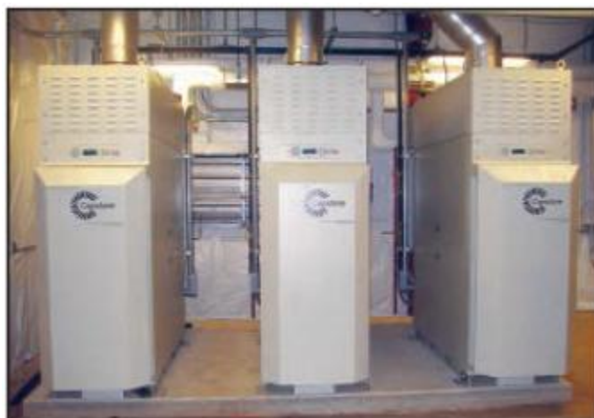
Fig 5.9: Through New Jersey's Public Utility Smart Start Incentive Program, the Salem Community College received a US$130 000 grant that helped fund the purchase of three Capstone natural gas C65 ICHP Micro Turbines.[3]
