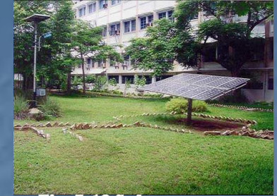
Fig. 5.13 Solar power generation
