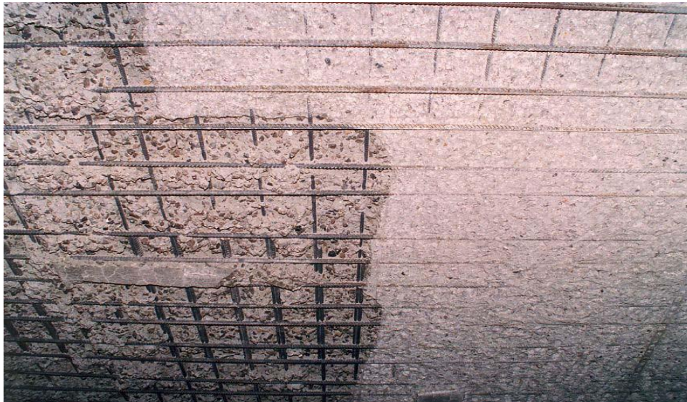
Fig:32 Spalling (expulsion) of the cover.
