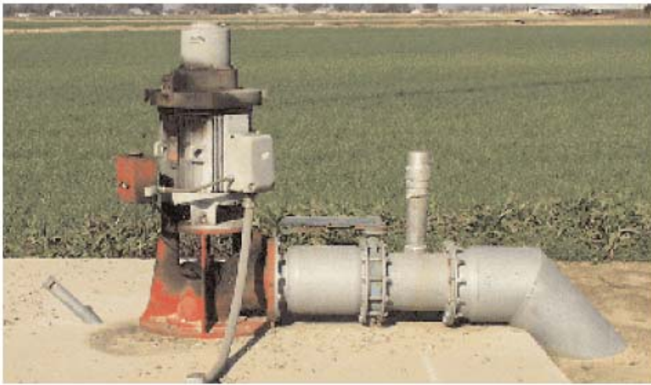
Figure 4.3: Properly completed well with elevated concrete seal (but with leaking lubricant).
