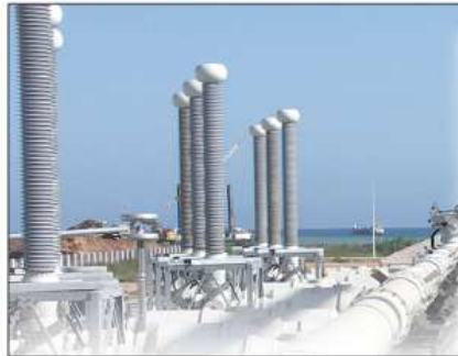
Power Generators (RBP)
