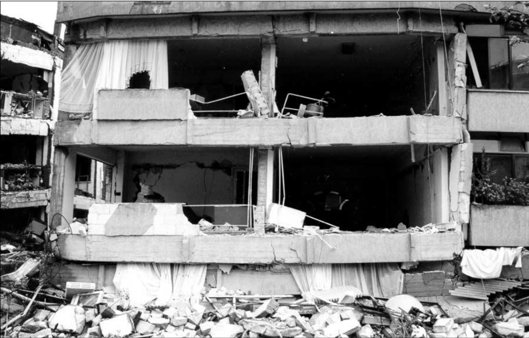
Figure 55 Examples of Failure due to Strong Beams and Weak Columns
