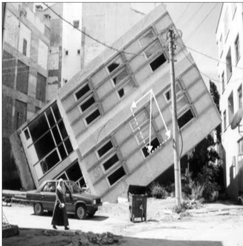
Figure 52 Foundation failure in 1999 Kocaeli Earthquake
