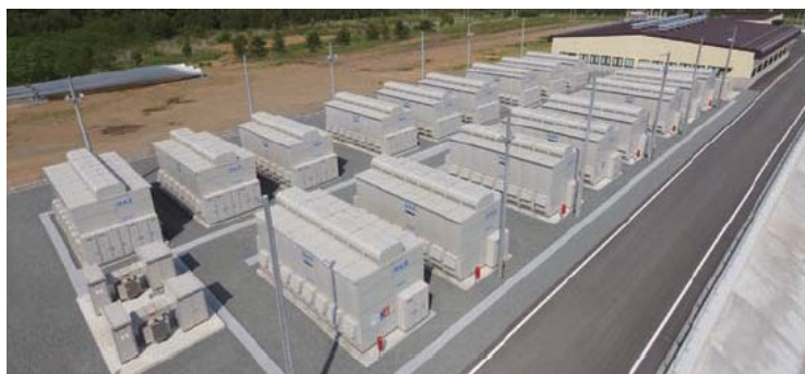
Figura 3.5 - Power system storage for wind-generator (Rokkasho village, Aomori)
