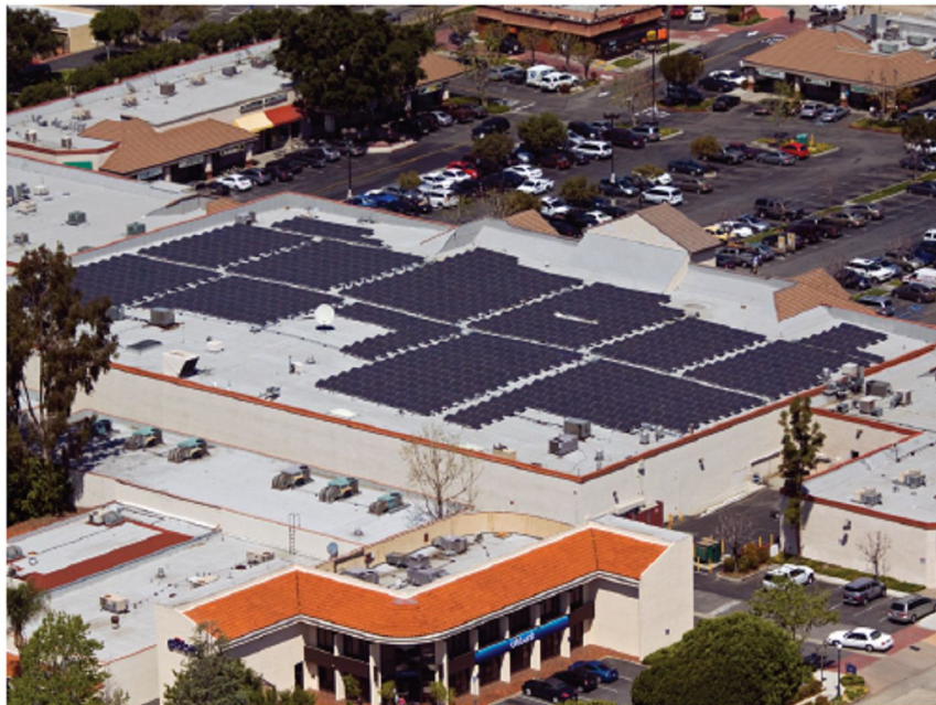
Figure 4.40: Photovoltaic system in a Grocery in Monrovia, California - SYSTEM SIZE: 230kW [ www.sunwize.com ]
