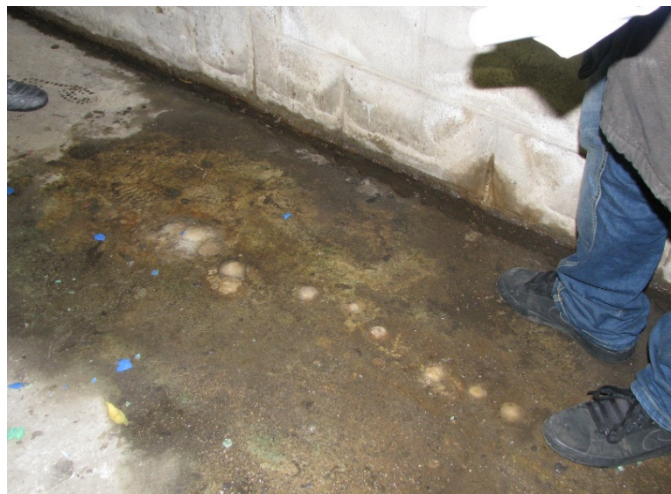
Figure 3-1 Water Flowing on the Floor
