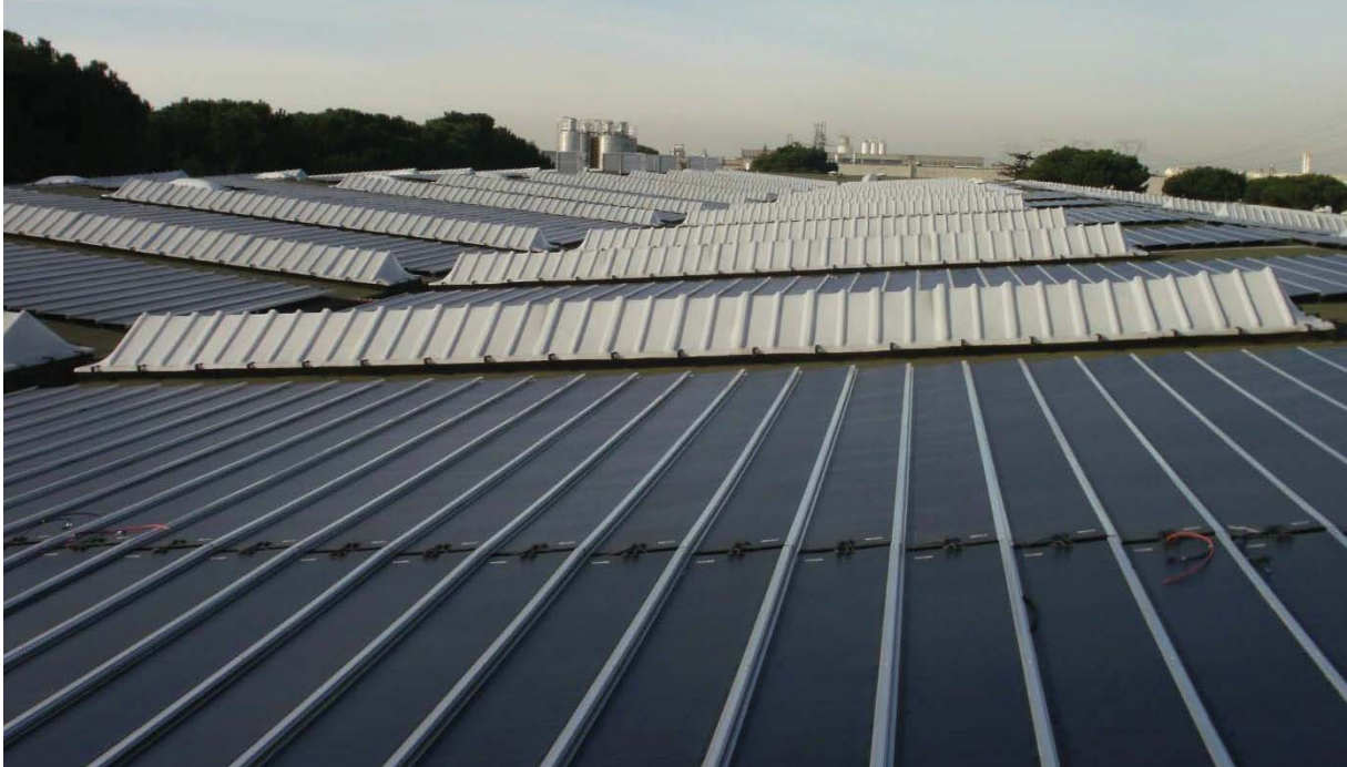
COCA-COLA HELLENIC BOTTLING COMPANY, ITALY SOLUTION FOR BITUMEN ROOF
