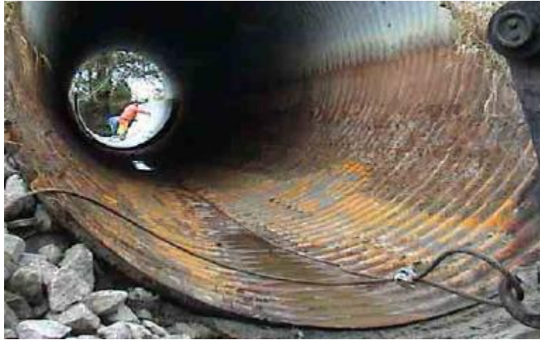
Figure 3.31 – Signs of corrosions in a cylinder culvert
