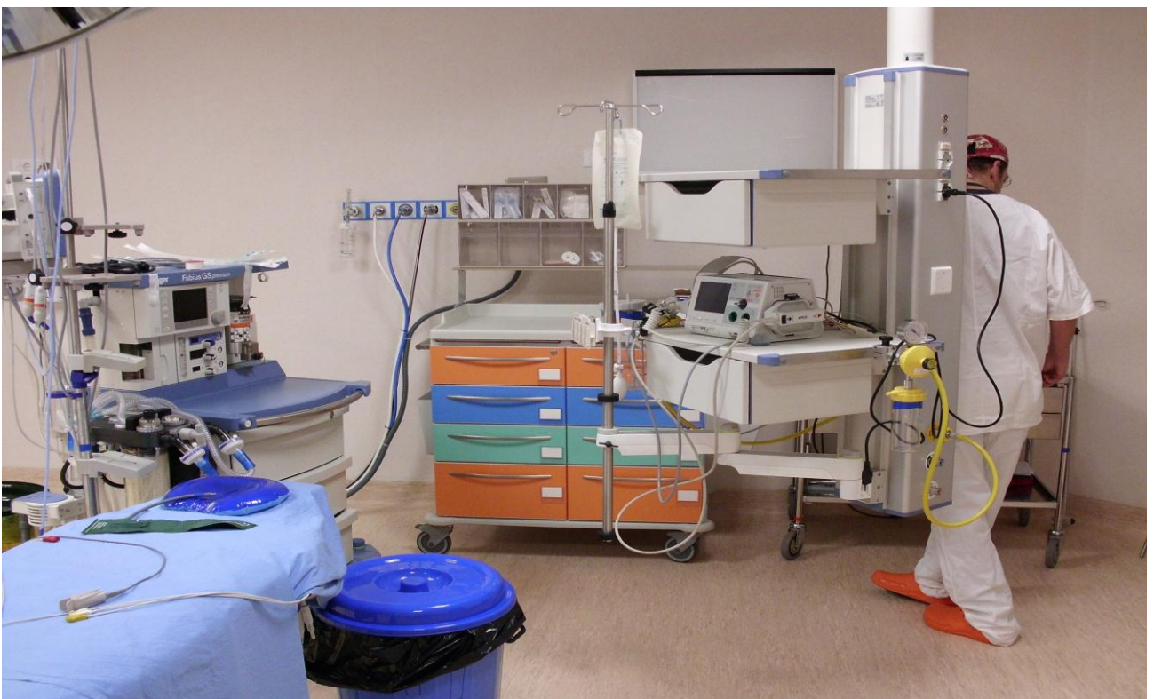
Fig.7: Operating Theatre (during equipment maintenance session) 2
