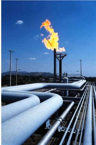
Figure 2.3: Gathering pipelines (source: Gazprom)
