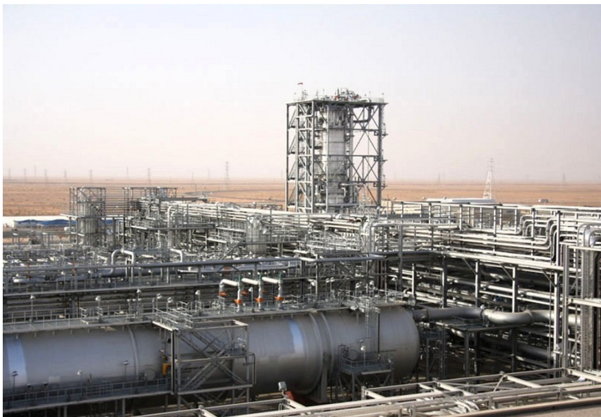
Figure 2.4: Gas oil separation plant (source: Saudi Aramco)
