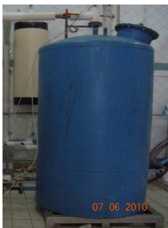
Figure 3-22 The PCM cold storage.
