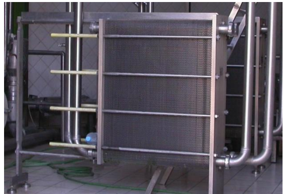
Figure 3-16 Heat exchanger used to cool the fresh milk arriving in the factory.
