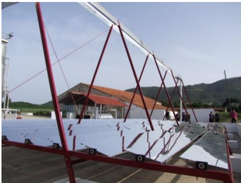
Figure 3-1 Fresnel solar thermal collector in the solar cooling system in Tunisia
