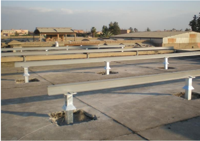
Figure 3-19 The supporting steel structure installed on the roof of the dairy factory.
