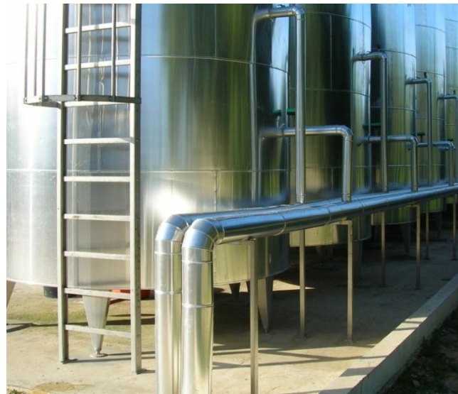
Figure 2-11 Fermenting tanks after insulation.
