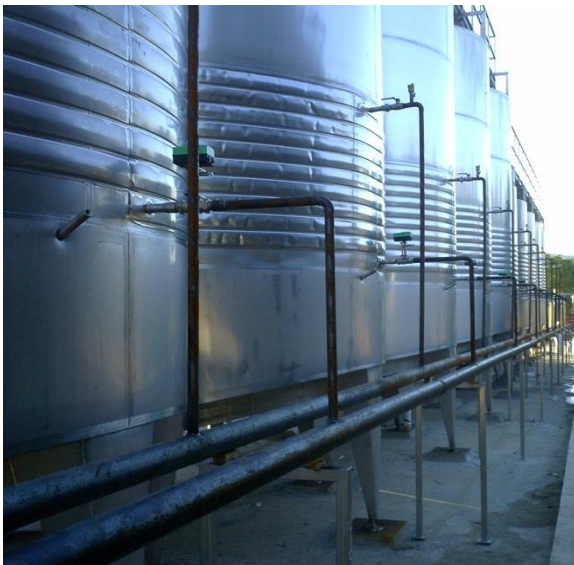
Figure 2-10 Fermenting tanks with chilled water circuit and jacket heat exchangers before insulation.
