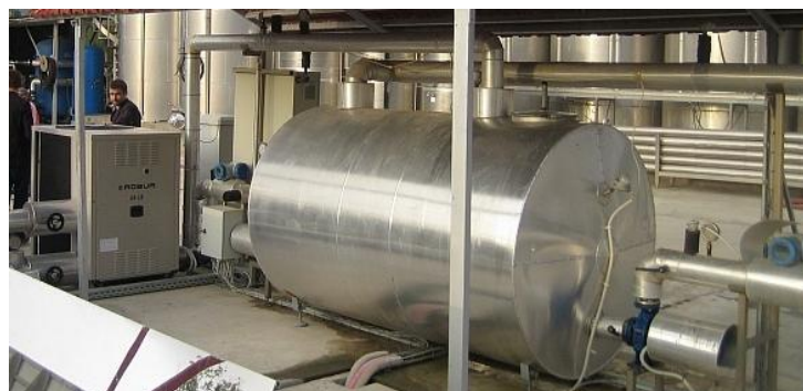
Figure 3-13 The installed cold storage.
