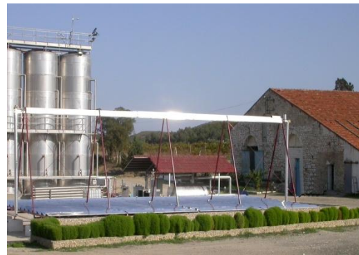
Figure 3-2 Fermenting tanks behind the installed solar thermal collector
