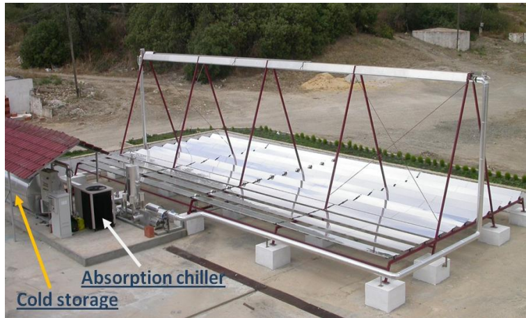
Figure 3-14 The first experimental setup, the solar collector, absorption chiller and cold storage.
