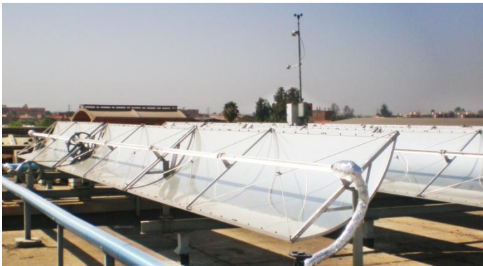
Figure 3-15 Parabolic trough collectors on the roof of the plant in Marrakech, Morocco.
