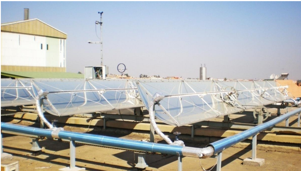
Figure 3-27 The parabolic trough collectors installed on the roof of the plant in Morocco.
