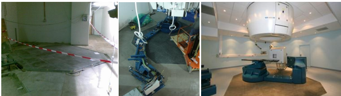
Figure 5.2 Installation of the systems in treatment room 1. From left to right: the pose of the granite floor, installation of PPS and PVS, a recent picture of the room acquired during accuracy tests.
