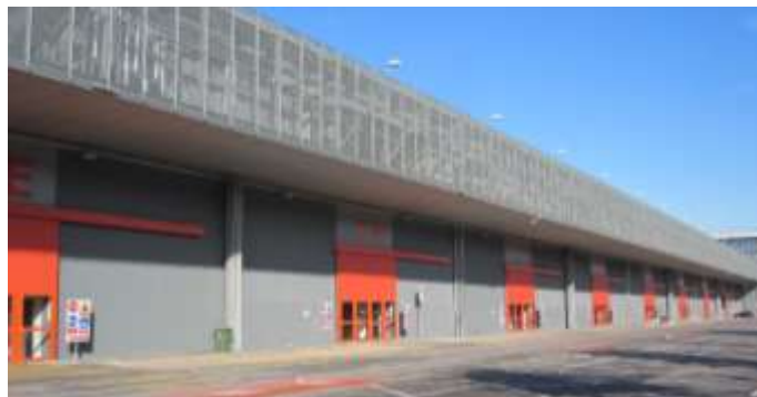
Figure 4-10. The main façade of the sample hall (east side, equal to west side).
