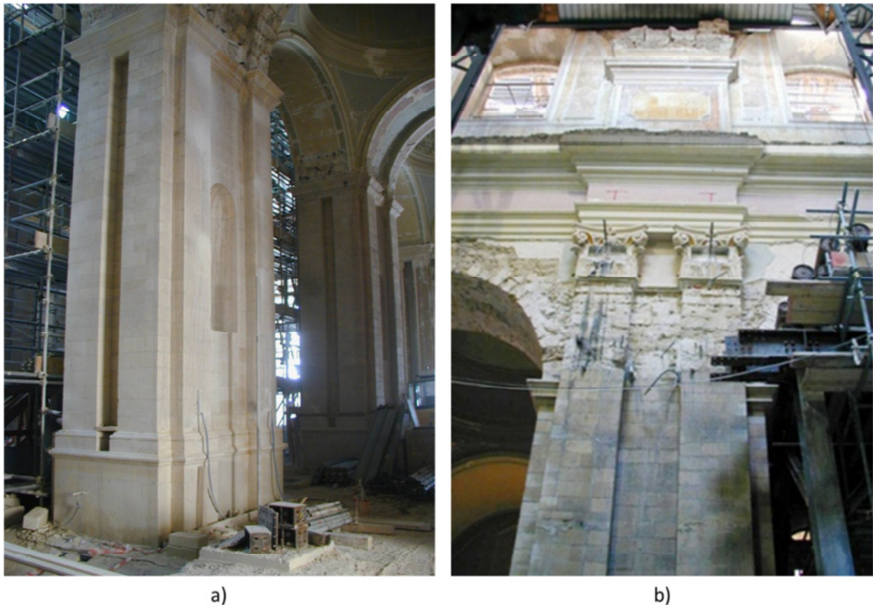
Figure 2.34: a) view of two pillars rebuilt from the basement to the springer; b) view of the connection between a rebuilt pillar and the overhanging original wall of the central nave of the cathedral (pictures by the author).
