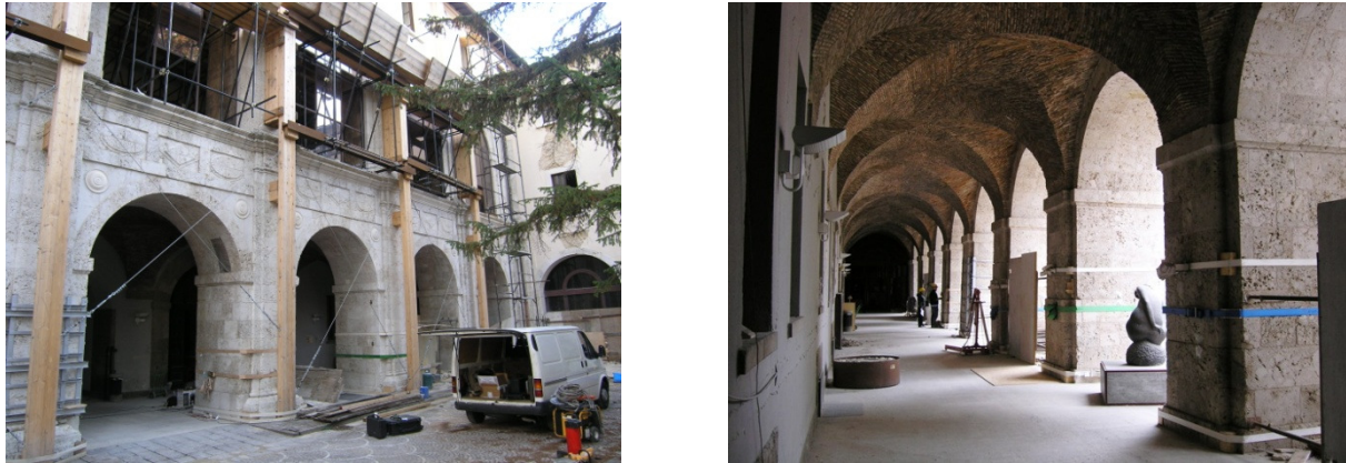
Figure 4.52: Views of the pilasters of the courtyard of the Spanish Fortress in L'Aquila (author's pictures).
