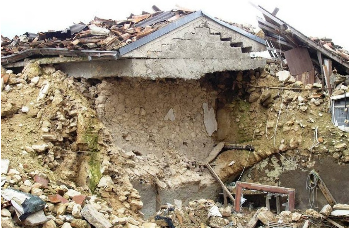
Figure 2.6: Onna (L'Aquila). View of a collapsed building, damaged by the wrong design of the new adapted r.c. roofing system, placed on the existing masonry structures (author's picture).
