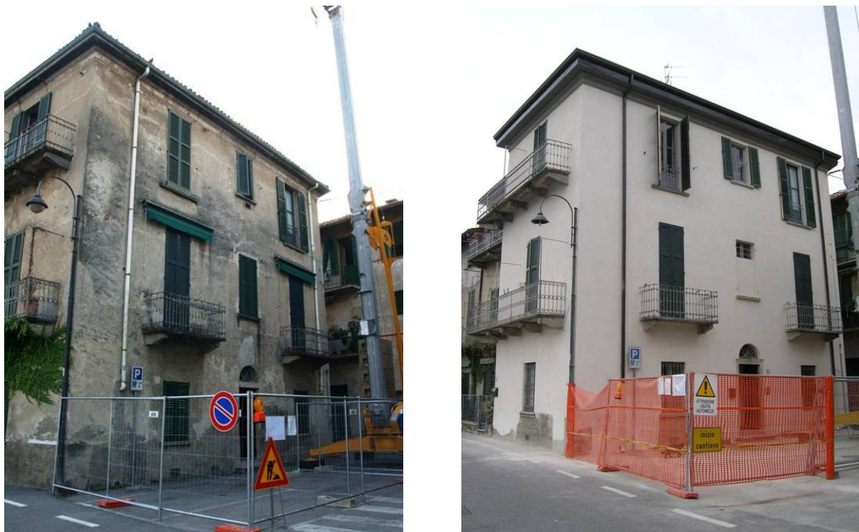
Figure 2.2: Views of the facade of a building in an historical centre before and after the renovation of the surfaces (author's picture).
