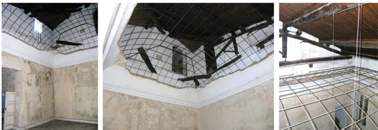
Figure 2.20: Reproduction of a collapsed vault in a room of Villa Borromeo-D'Adda in Arcore (Milan), a misused building under the protection of the FAI - Italian Fund for the Environment (pictures by the author).
