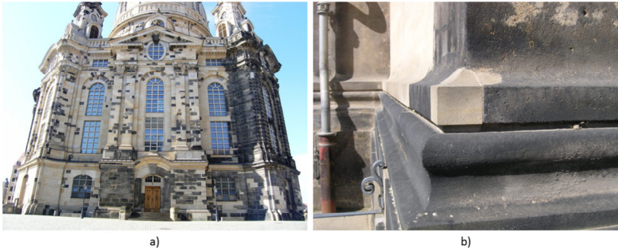
Figure 2.23: a) South front of the Fraenkirche in Dresden; b) detail of the integration of a moulding, maintaining the original material (pictures by the author).
