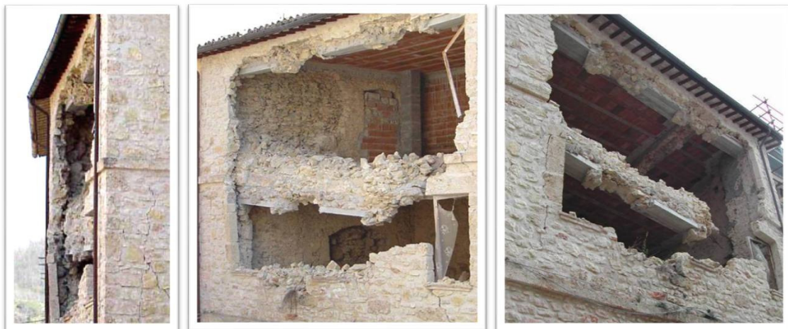
Figure 1.23: Three views of a building stroke by the 1998 Umbria earthquake. The overturning of the façade is connected to the presence of stiff floors made by hollow bricks and reinforced concrete (courtesy of Arch. Antonella Saisi).
