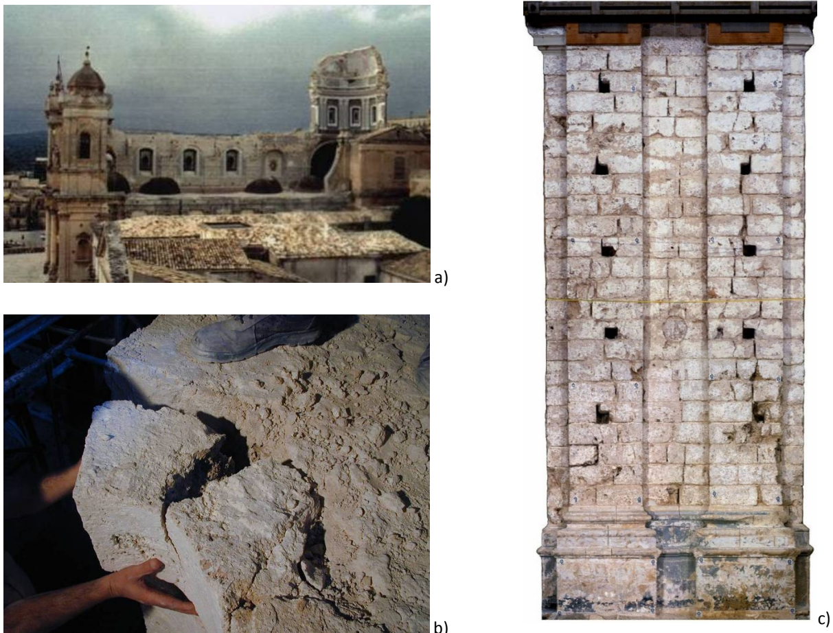
Figure 2.5: Pictures from the collapsed Noto Cathedral: a) view of the interior of the cathedral after the collapse (picture taken from R. De Benedictis e S. Tringali "La ricostruzione della Cattedrale di Noto", LCT Edizioni, 2000, p. 20 (De Benedictis, 2000)) ; b) view of a stone during the dismantling of a pilaster (courtesy of prof. L. Binda); c) digital photo-straightening of one side of a pillar of the nave after the removal of the plaster (courtesy of A. Saisi).
