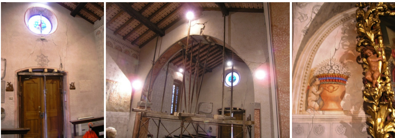
Figure 4.43: Views of the main cracks in a church damaged by the earthquake in the Garda Lake area (pictures by the author)
