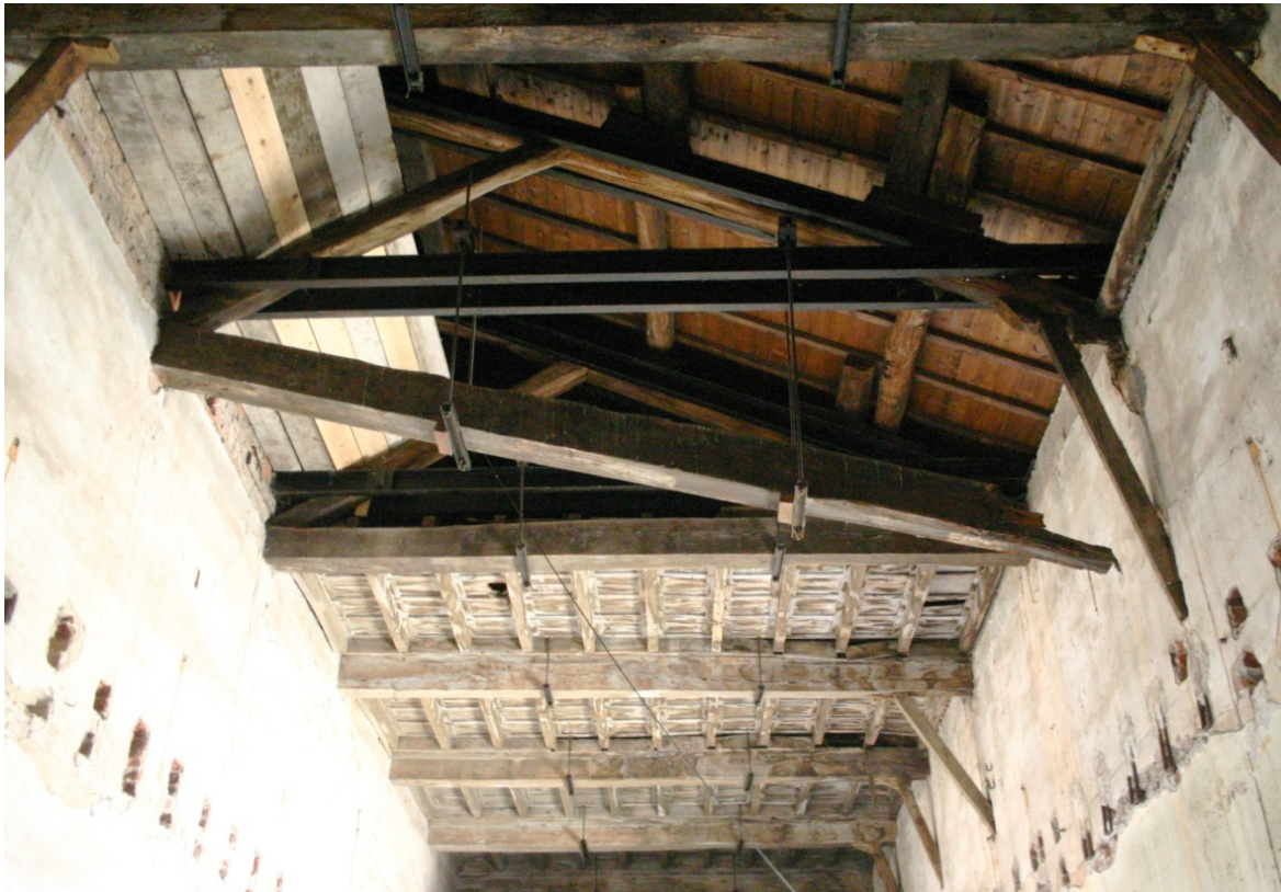
Figure 2.21: Example of a didactical arrangement of a collapsed truss in a room of the Melegnano Castle (Milan), substituted by a steel beam (picture by the author).
