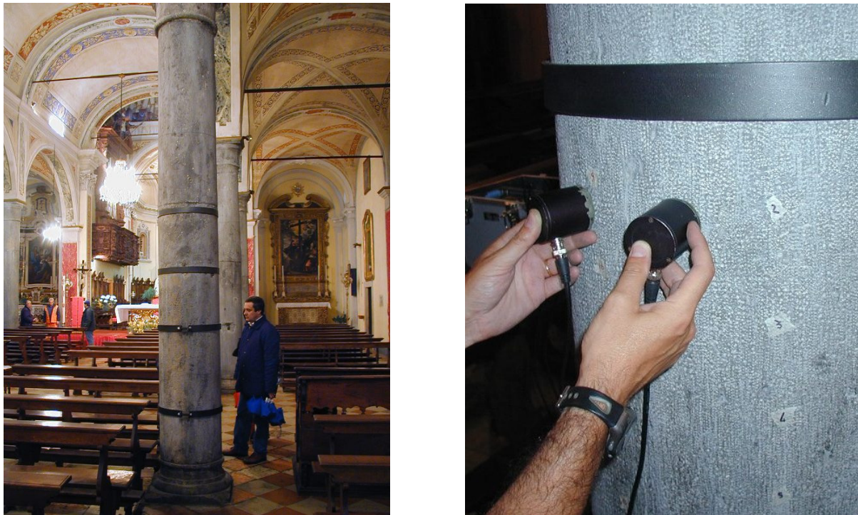
Figure 4.47: View of the damaged column, presenting a diffused crack pattern and application of the transducers for the ultrasonic test (author's pictures).
