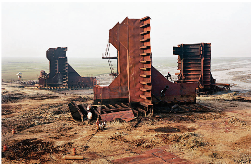
Edward Burtynsky Shipbreaking # 27, With Cutter, Chittagong, Bangladesh 2000
