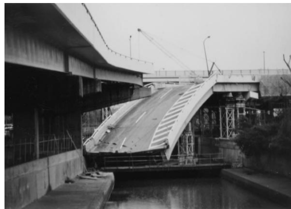
Figure 1.5. Example of damaged bearing and collapsed span, 1995 Kobe earthquake [10]
