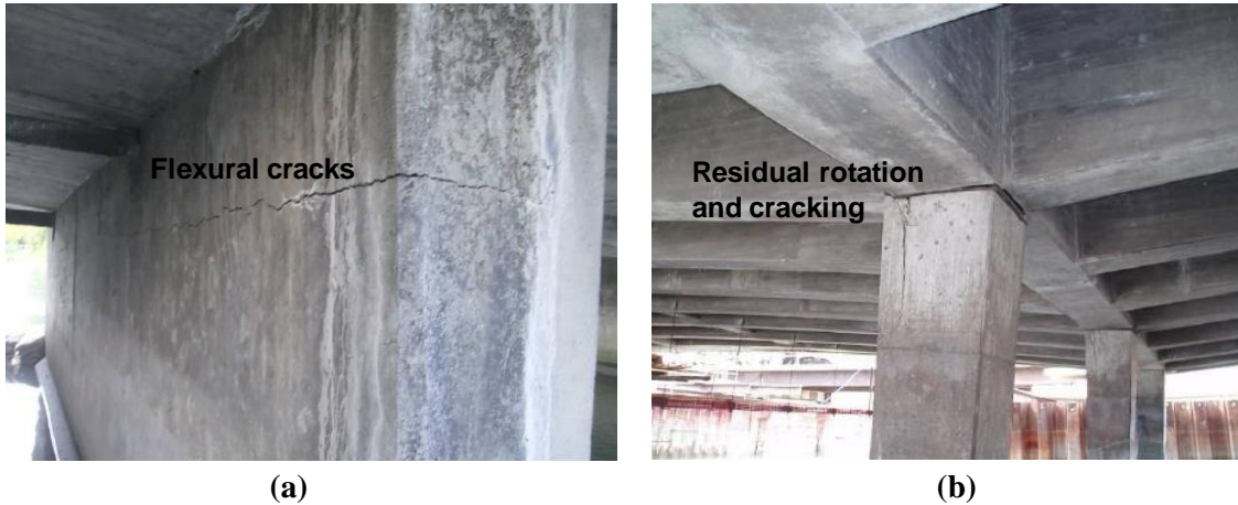
Figure 2.10. a) Damaged pier in Gayhurst Road Bridge [Photo by L. Hogan]; b) Cracked and rotated piers of Ferrymead Rd. Bridge [Photo from CCC]
