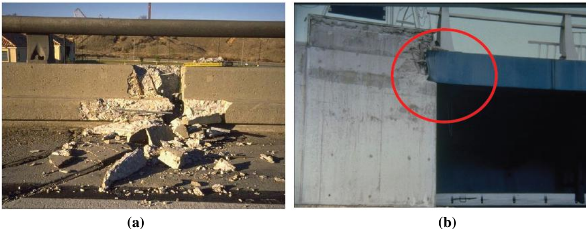
Figure 1.11. Pounding damage: (a) between adjacent spans at the Interstate-5 at Santa Clara River in Los Angeles County during the 1994 Northridge earthquake and (b) at the abutment of a bridge near Nishinomiya Port in the 1995 Kobe earthquake [8]
