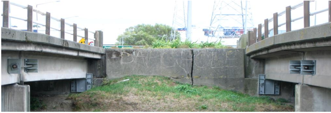
Figure 5.10. Transverse crack at the northwest abutment
