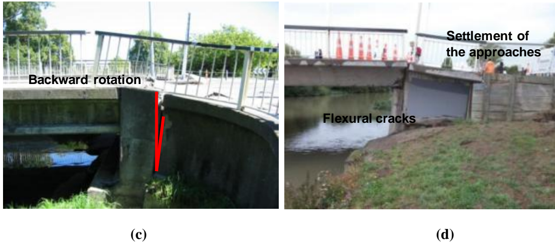
Figure 2.7. Damage at the abutments: a) Sketch of the forces acting on abutments and foundations in undeformed condition; b) Back rotated abutments of Fitzgerald Bridge [Courtesy of OPUS]; c) Back rotated abutments of Bridge Street Bridge [Photo by M. Bruneau]; d) Damaged abutments of Avondale Road Bridge [Courtesy of OPUS]
