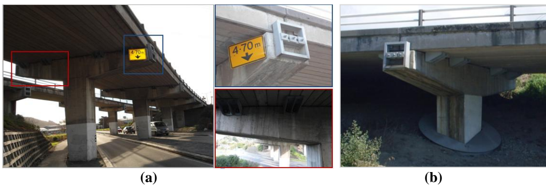
Figure 4.2. Retrofit solutions fitted to the bridge (a) Shear keys and pier linkages; (b) Circular steel shroud
