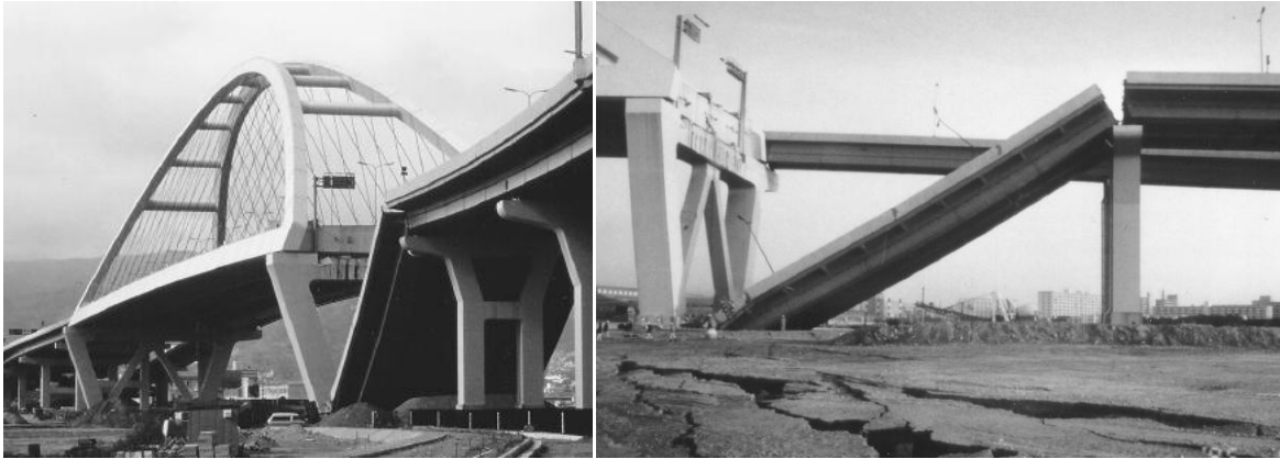
Figure 1.8. Unseating of simply supported link span, Nishinomiya-ko bridge, Kobe earthquake
