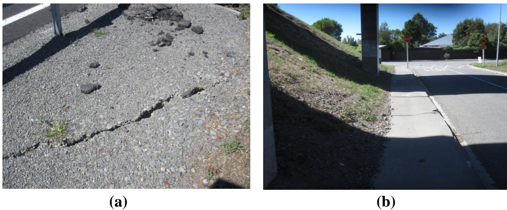
Figure 5.6. a) Cracks on the top of the embankment; b) Cracks in the pavement under the bridge
