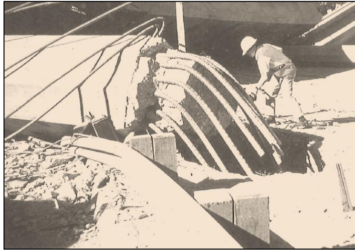
Figure 1.23. Pullout failure, 1971 San Fernando earthquake [7]
