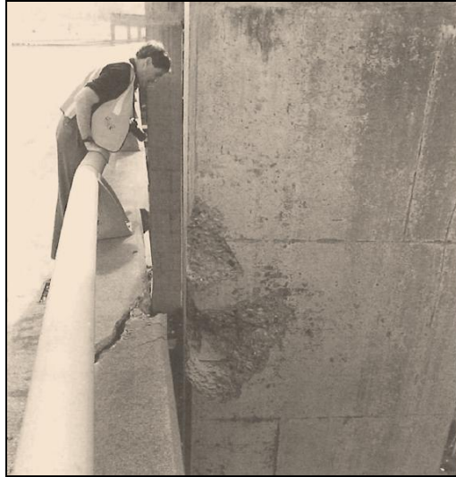
Figure 1.10. Pounding of I-280 China Basin/Southern viaduct, 1989 Loma Prieta earthquake [7]
