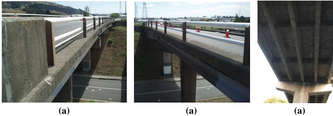
Figure 5.3. (a-b) General view of the superstructure and (c) deck soffit of the bridge
