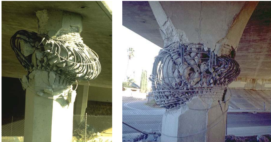
Figure 1.18. Confinement failure at bridge pier top, 1994 Northridge earthquake [8]
