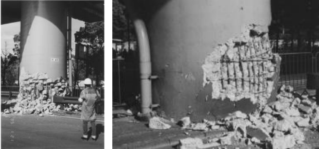
Figure 1.15. Two examples of flexural failure due to lack of confinement at bottom of reinforced concrete piers supporting a steel superstructure, 1995 Kobe Earthquake [10]
