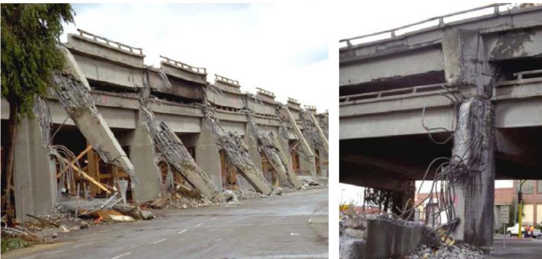
Figure 1.21. Sliding shear at top columns of the Cypress viaduct in the 1989 Loma Prieta earthquake [8]
