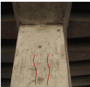
Figure 6.8. Pier 3, south column, fine vertical cracks at the top and horizontal flexural cracks.
