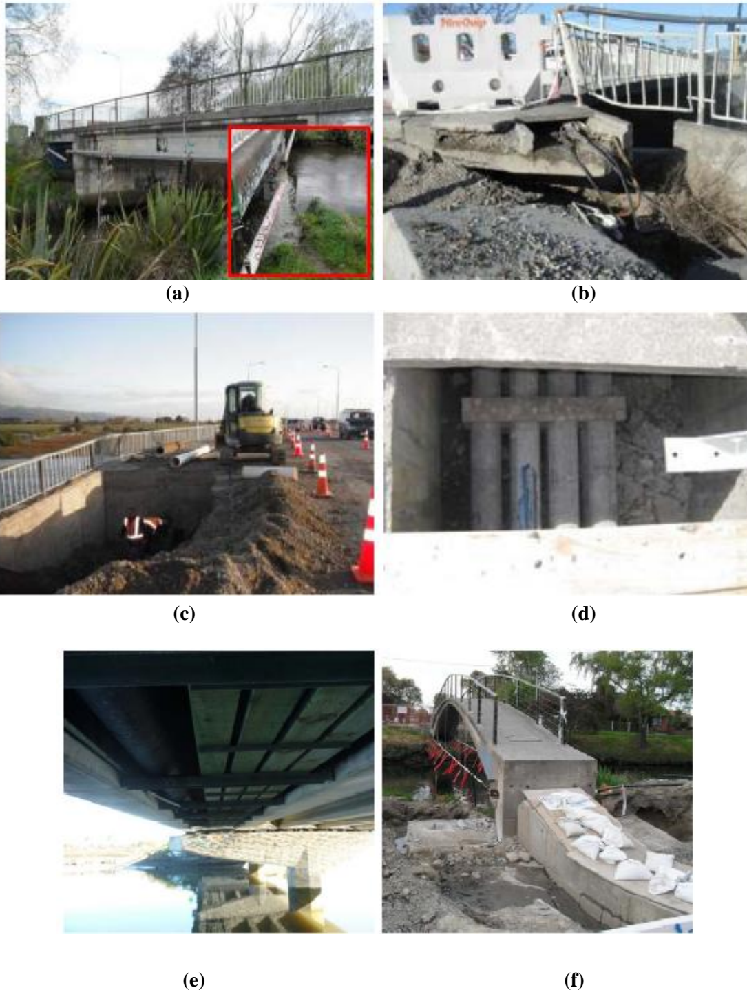
Figure 2.18. a) Damage to pipelines at Kainga Road Bridge after September 4, 2010 [Photo by A. Palermo]; b) Gayhurst Road Bridge: damage to lifelines [Photo by A. Palermo]; c) Repairing works at at Bridge Street Bridge [Photo by A. Palermo]; d) Close-up view of damaged pipes along the deck of Ferrymead Bridge [Courtesy of OPUS] e) Damaged pipelines at Bridge Street Bridge after June 13, 2011 [Photo by E. Camnasio]; f) Dallington Pedestrian Footbridge: damage to electrical services to the Dallington area [Photo by M. Le Heux]
