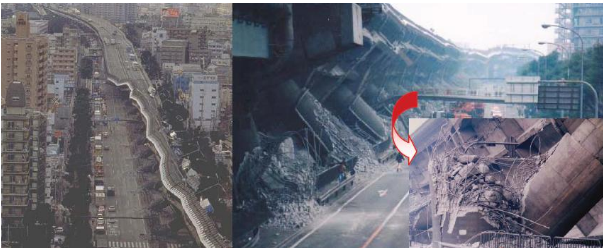
Figure 1.16. Flexural failure above column base of columns of the Hanshin expressway, due to premature termination of longitudinal reinforcement and inadequate confinement in the 1995 Kobe earthquake [8]
