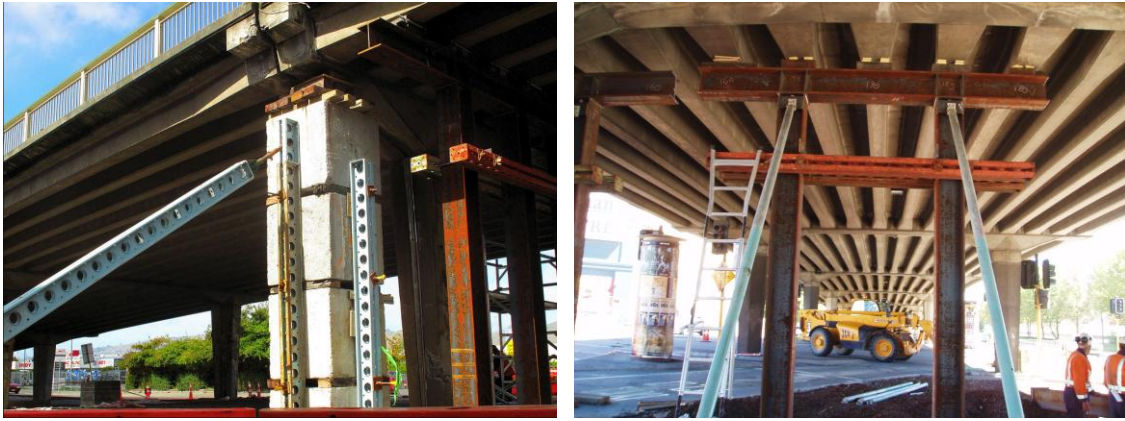
Figure 6.13. Temporary strengthening at failed pier at date of inspection (22/03/11).
