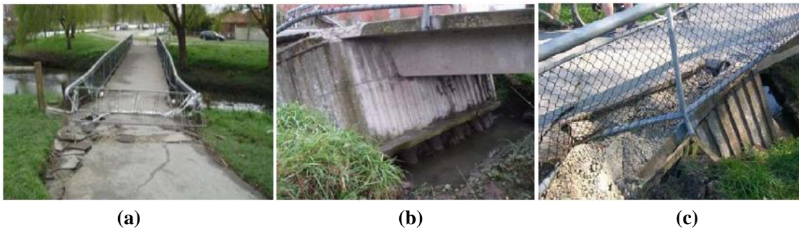
Figure 2.16. Porritt Park Pedestrian Bridge: a) End view [Photo courtesy of OPUS International Ltd]; b) Backward rotation of abutment and exposure of piles [Photo courtesy of OPUS International Ltd]; c) Repairing damage to approach and river bank lateral spreading [Photo by L. Hogan]
