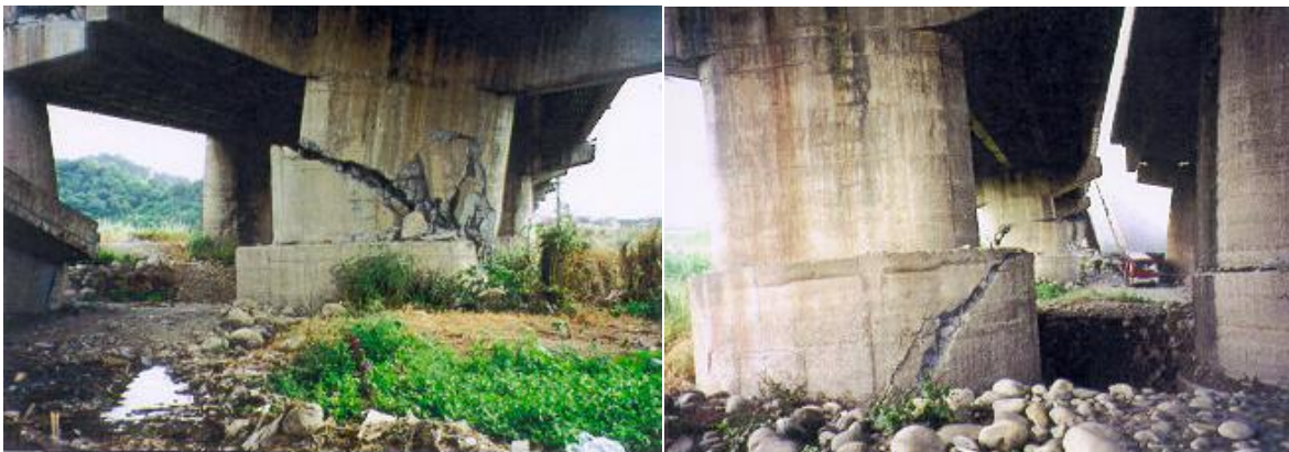
Figure 1.19. Wushi Bridge, shear failure of piers P2S and P3N, 1999 Taiwan earthquake [9]
