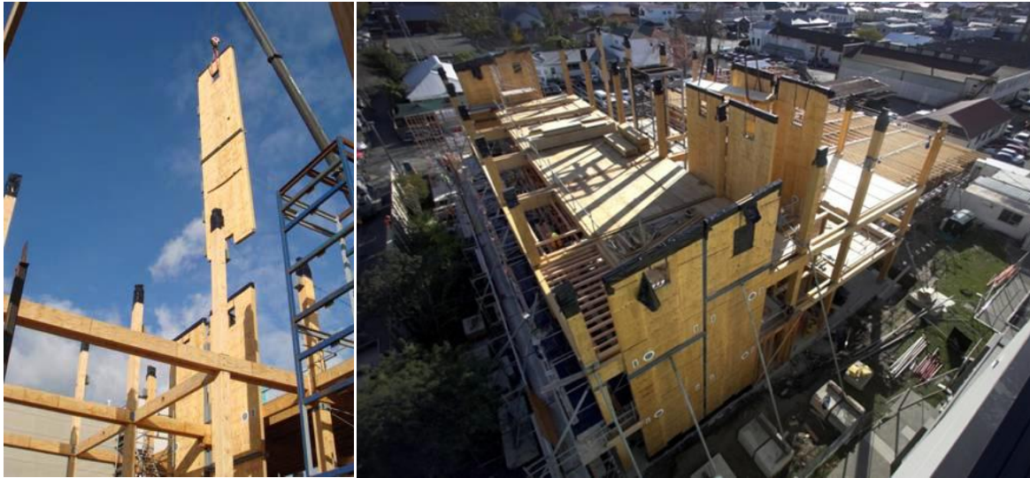
Figure 180. Photos taken during construction and installation of LVL post-tensioned and coupled shear panels, NMIT Arts & Media Building
