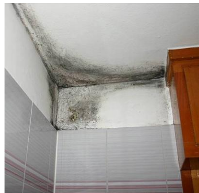
Figure 2.9 - Superficial condensation photo [W11]
