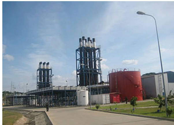
Figure 4.18.: Ubungo gas plant
