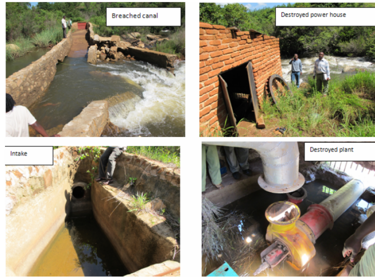
Figure 22.15.: Mpando, failed plant equipment
